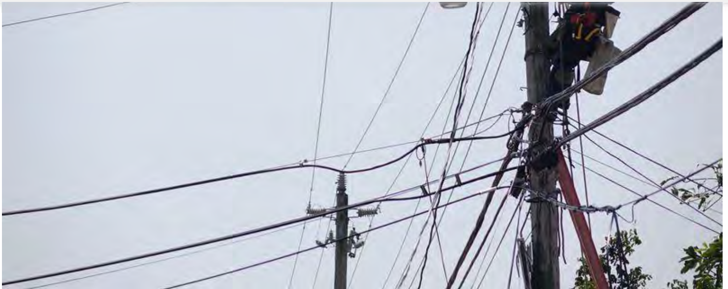
A lineman with Florida Power and Light works on connecting a residence in Oakland Park after 2017's Hurricane Irma. (JOE CAVARETTA / Sun Sentinel)
