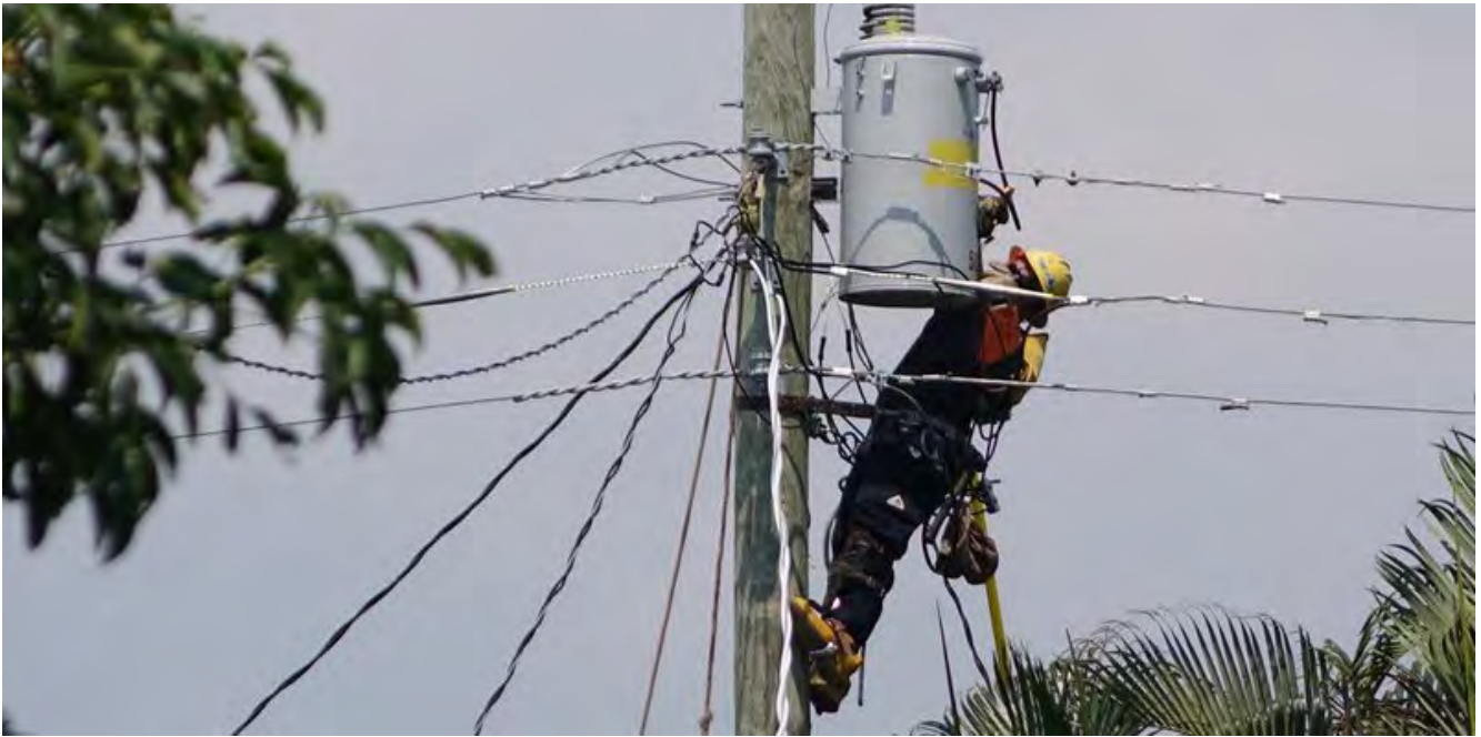
A lineman working with Florida Power and Light replaces a transformer in Oakland Park after Hurricane Irma. (JOE CAVARETTA / Sun Sentinel)
