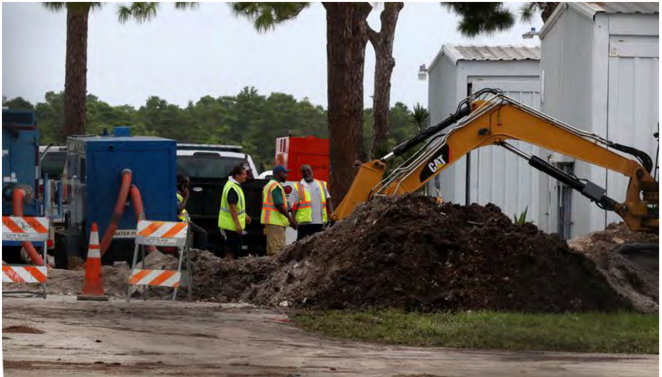
Florida Communication Concepts Inc. was repairing electric lines for Florida Power & Light in the 2500 block of Northwest 55th Court when the water main was struck and damaged, Fort Lauderdale Mayor Dean Trantalis said in a statement. (Carline Jean / South Florida Sun Sentinel)
