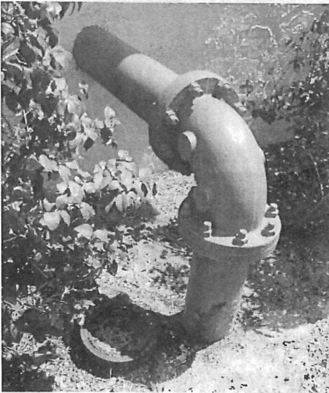
Figure 3. Corrosion observed on pipe leading from pump house for well#1.
