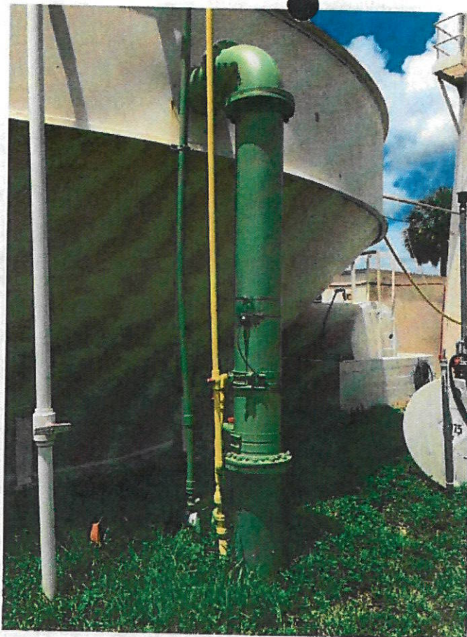
FIGURE 7. RAW WATER RISER METER TEST AREA WIRE BRUSHED AND ANTI CORROSION COATED.
