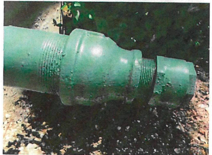
FIGURE 4. CORROSION ON FLUSH-LINE WELL #1. FITTING TIGHTENED, WIRE BRUSHED, ANTI CORROSION COATED.
