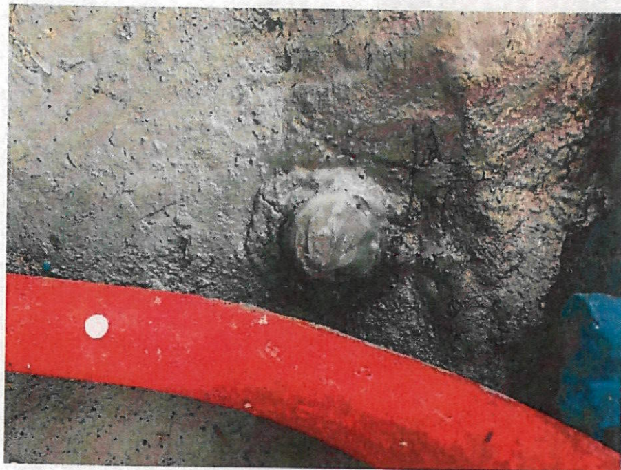
FIGURE 8. HS PUMP #2 DEAD WIRES IN ABANDONED CONDUIT SEALED & COATED.
