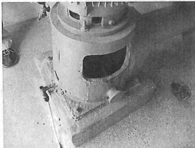
Figure 7. Corrosion observed at the head of well#3.
