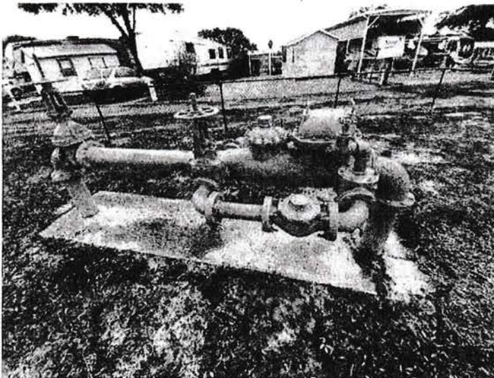
Meter at Fawn Ridge:
