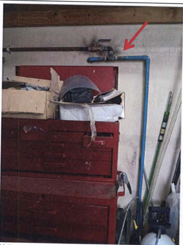
Make-up water line for fluoride.
