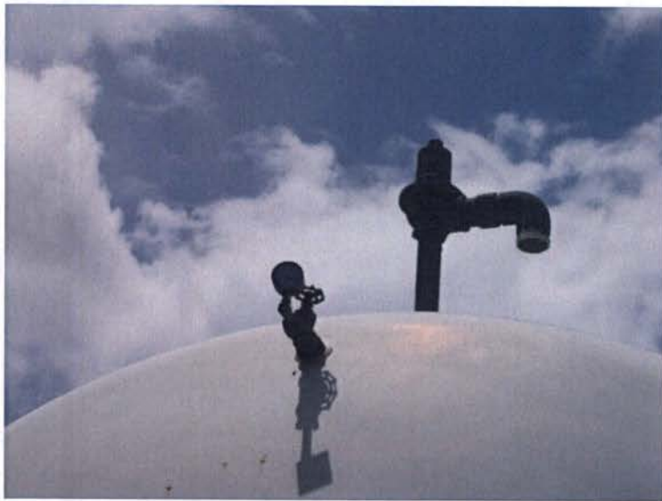
Figure 15. New pressure gauge installed on hydro tank.
