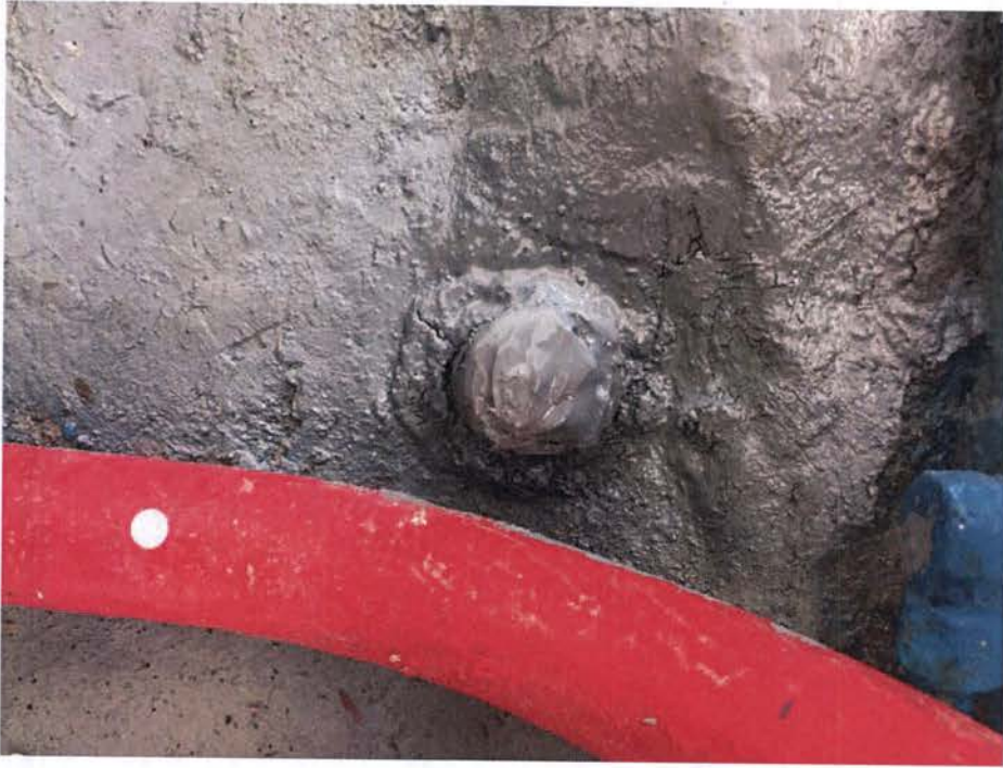
FIGURE 13. HS PUMP #2 DEAD WIRES IN ABANDONED CONDUIT SEALED & COATED.
