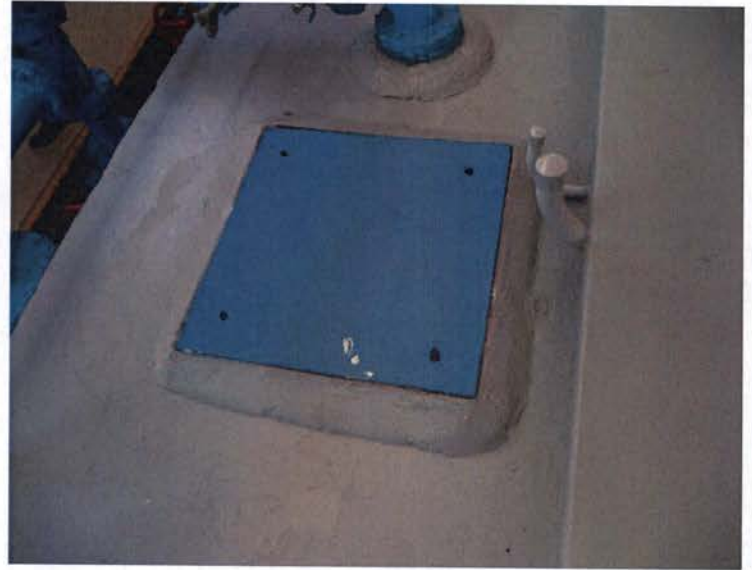
Figure 2. A plate with four (4) small holes was observed on top of the clearwell.
