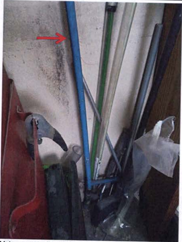
Make-up water line for fluoride.
