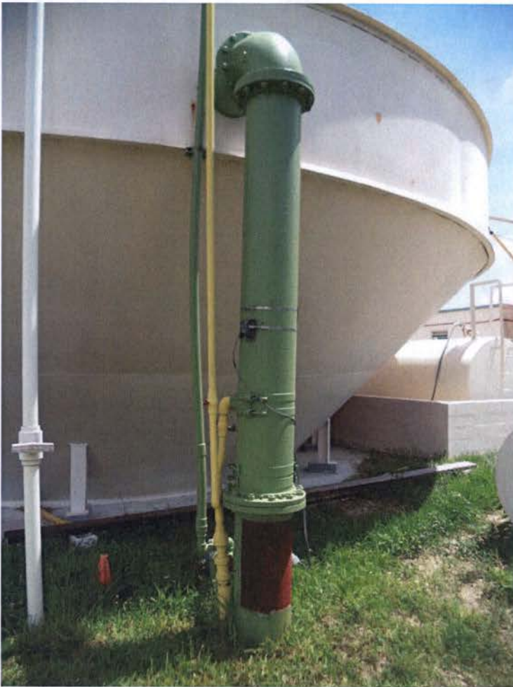
Figure 9. Corrosion on manifold pipe leading to Accelerator.
