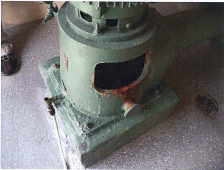
Figure 7. Corrosion observed at the head of well#3.
