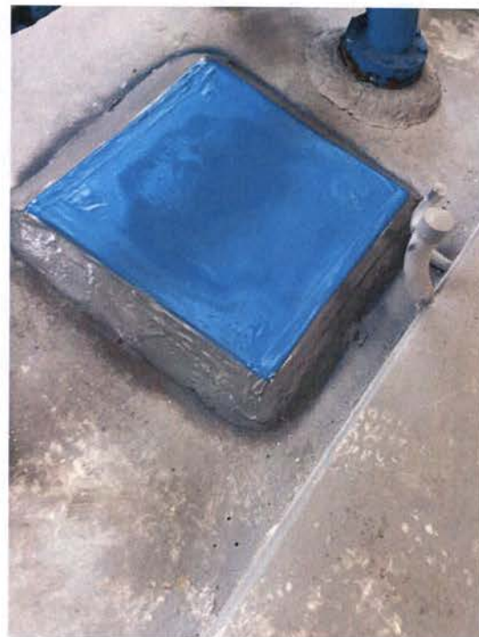
FIGURE 2. POSITION FOR FUTURE BWT #2 SEALED.
