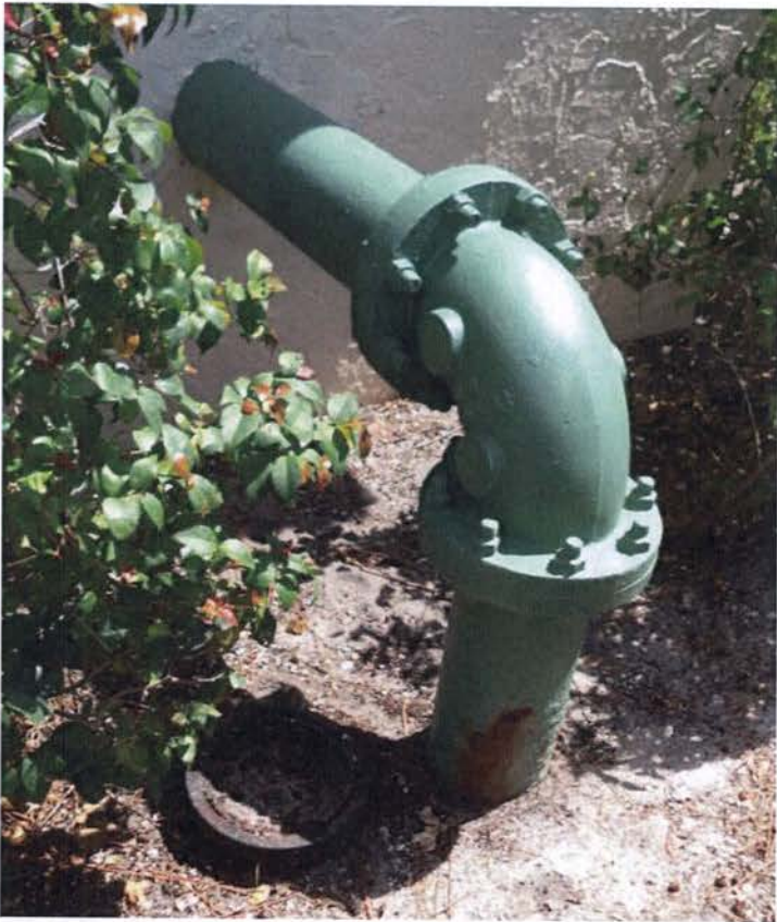
Figure 3. Corrosion observed on pipe leading from pump house for well#1.
