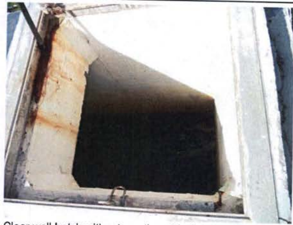
Clear well hatch without weather stripping
