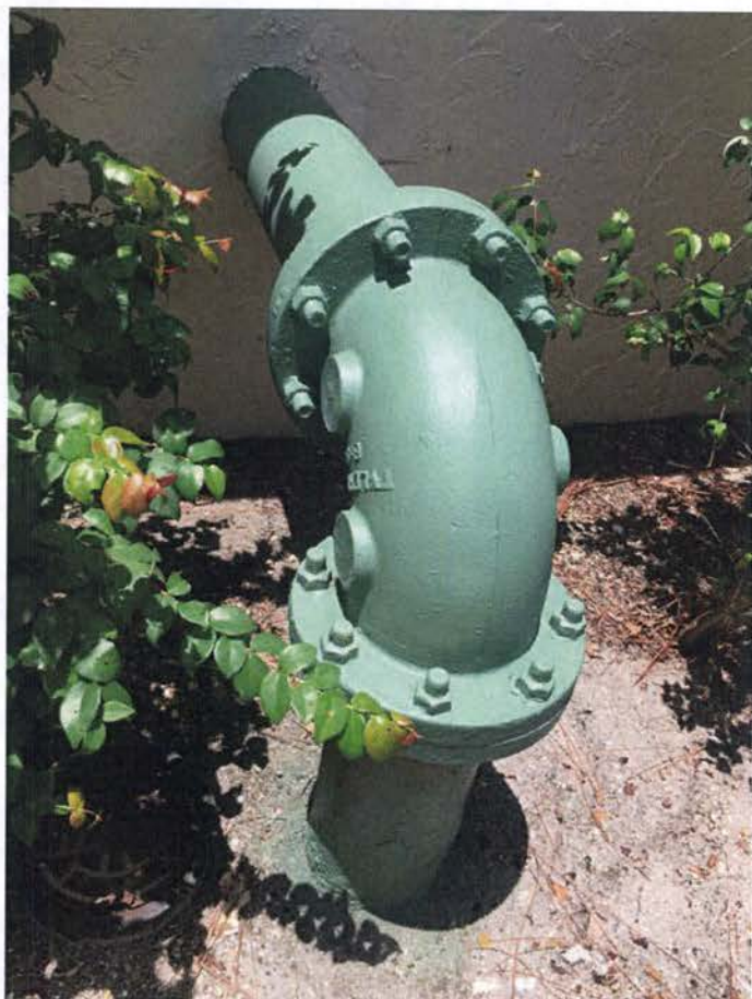
FIGURE 3. CORROSION ON WELL #1 DISCHARGE PIPE WIRE BRUSHED, ANTI CORROSION COATED.
