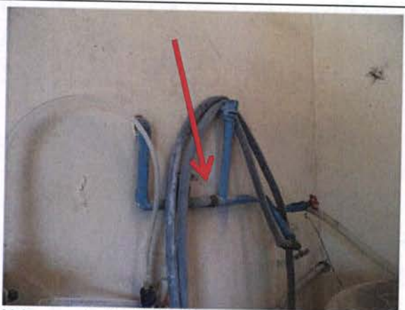
Make-up water line for fluoride.
