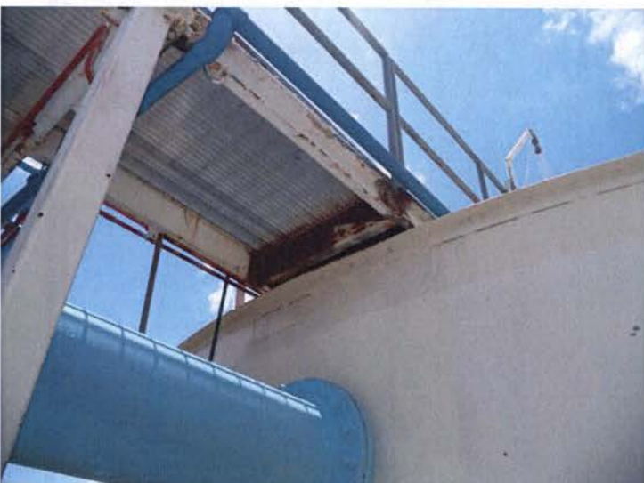
Figure 11. Corrosion on the underside of walkway leading to Accelerator.
