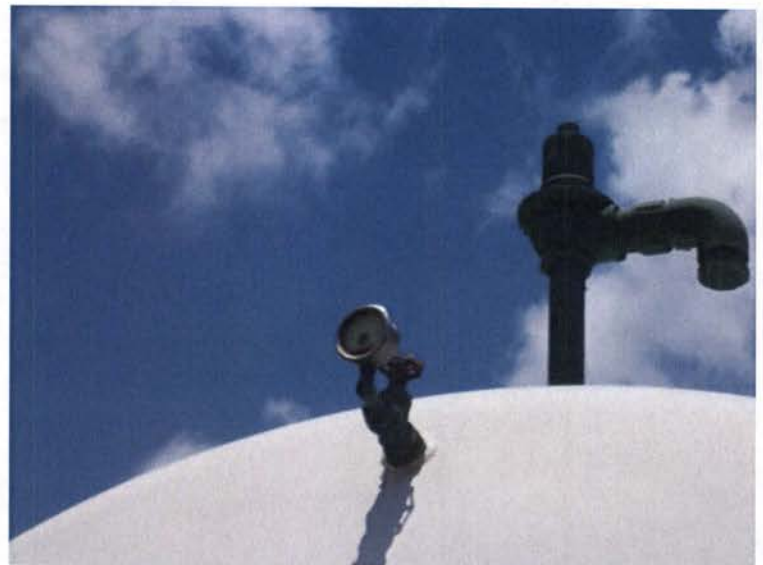
Figure 14. Broken pressure gauge on the hydro tank (Corrected next day, see figure 15).
