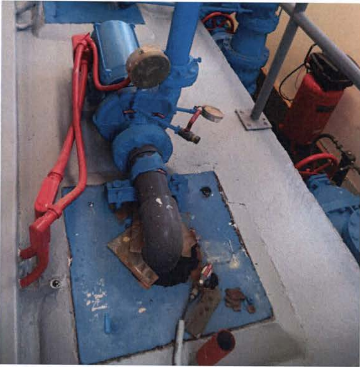
Figure 1. Hole observed in top of the clearwell.
