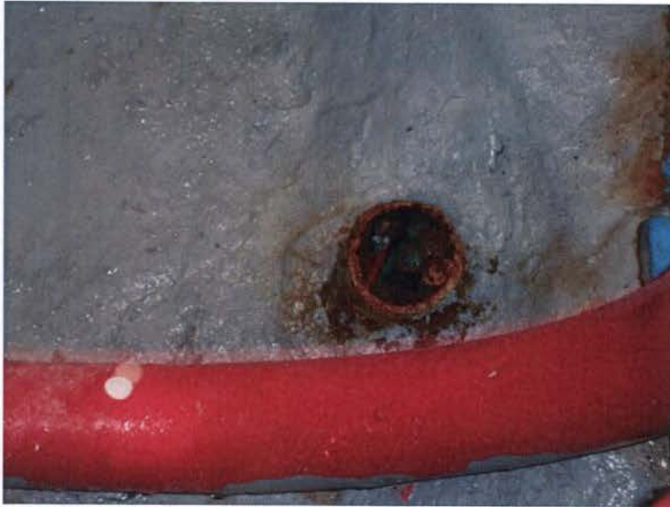
Figure 13. Exposed electrical wiring near the high service pumps. This is not found as a deficiency because they are not electrically active and the conduit is plugged; however, it is recommended to cap or otherwise cover the exposed wires.
