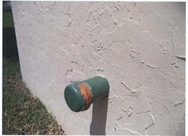
Figure 8. Corrosion on flush-line cap at well#3.
