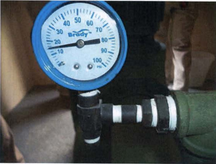
Figure 5. Broken pressure gauge at well#2 (corrected on site, see figure 6).
