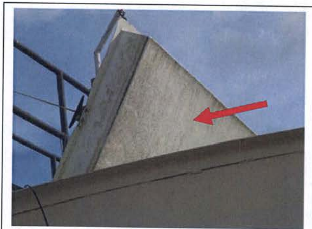
Biogrowth on clarifier's boat.
