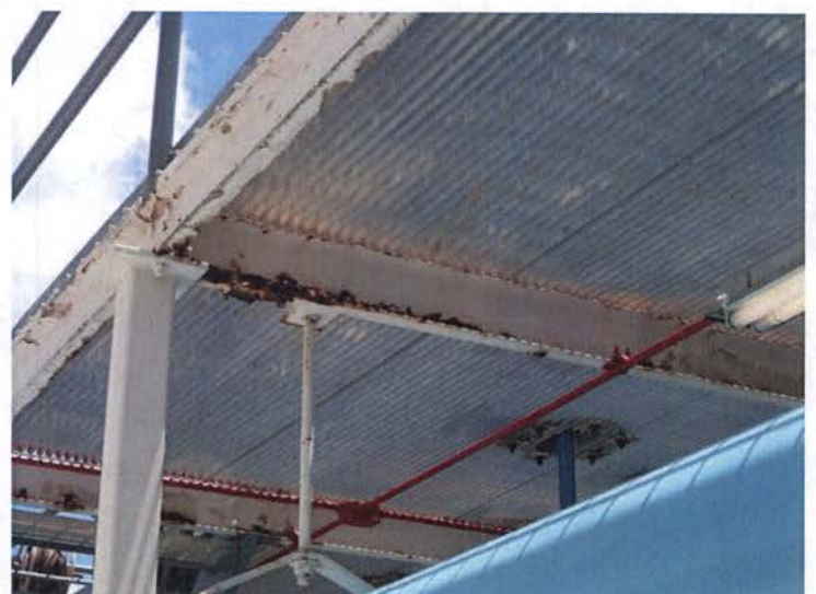
Figure 12. Corrosion on underside of walkway leading to Accelerator.
