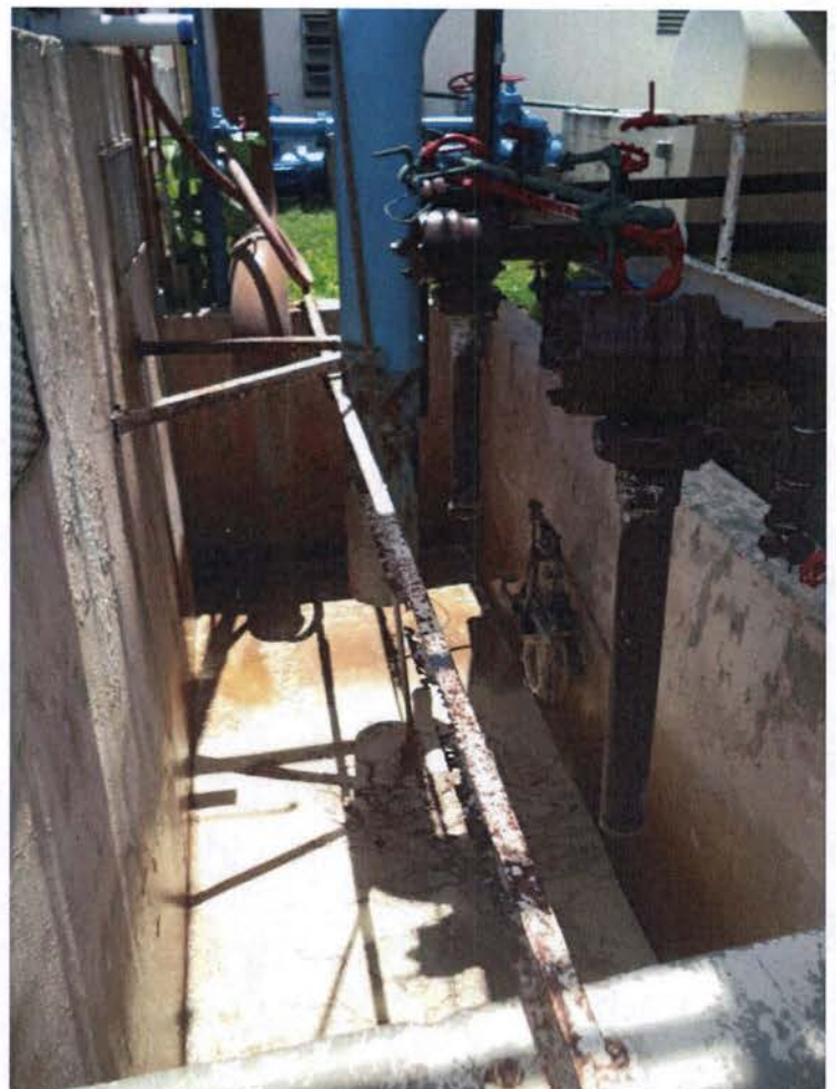
Figure 10. Corrosion on pipe at the sludge collector tank.
