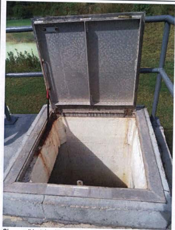
Clear well hatch without weather stripping.
