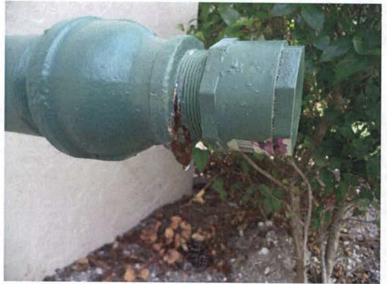
Figure 4. Corrosion and leak observed at the flush-line cap for well#1.
