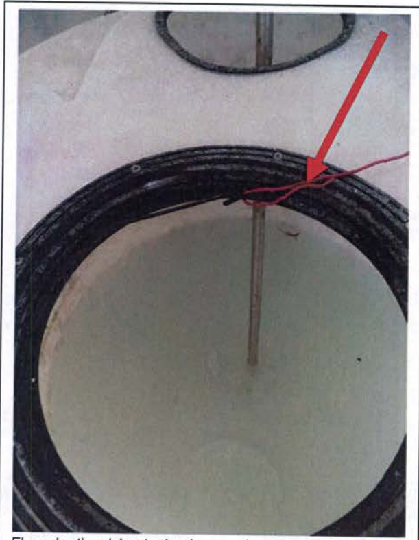
Flocculant's mixing tank w/exposed opening.
