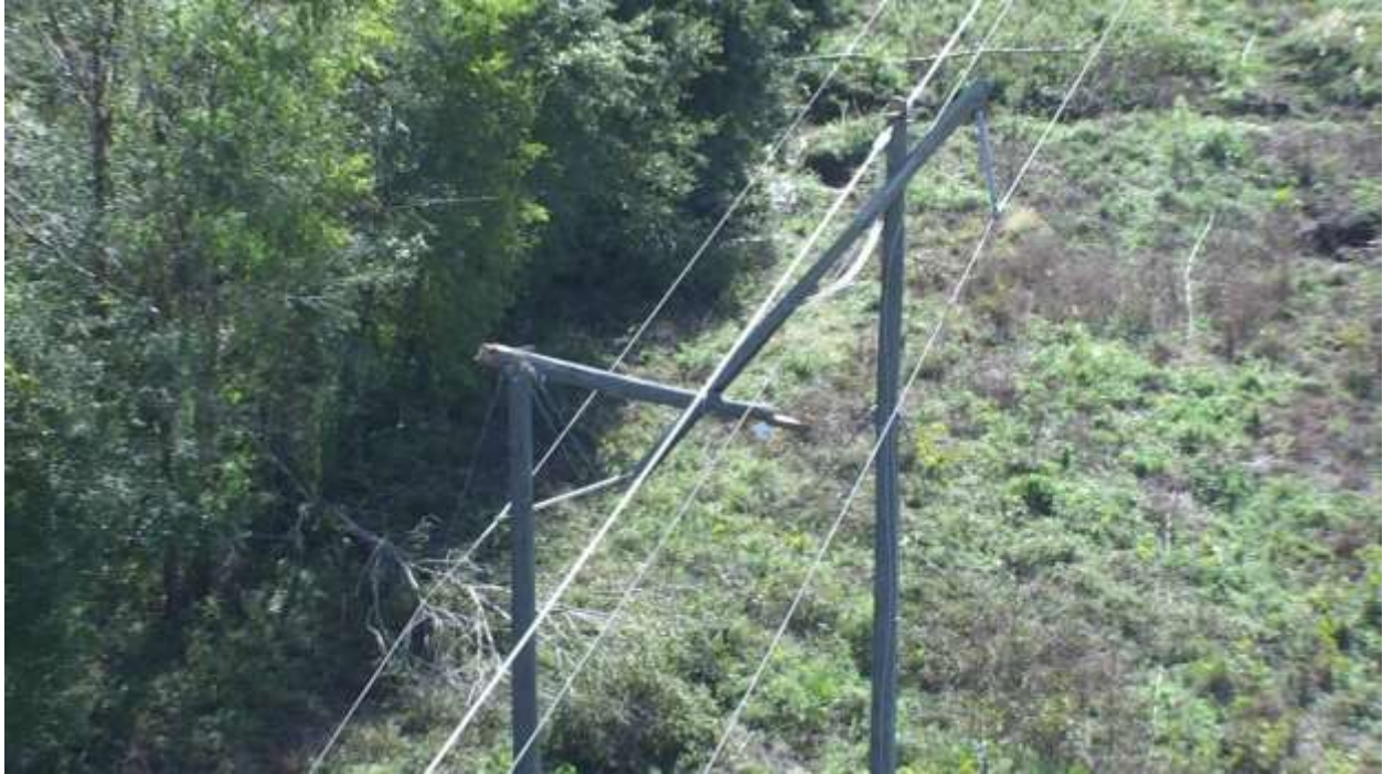
FIGURE 5 – WOOD POLE FAILURE AT STORM GUYS
