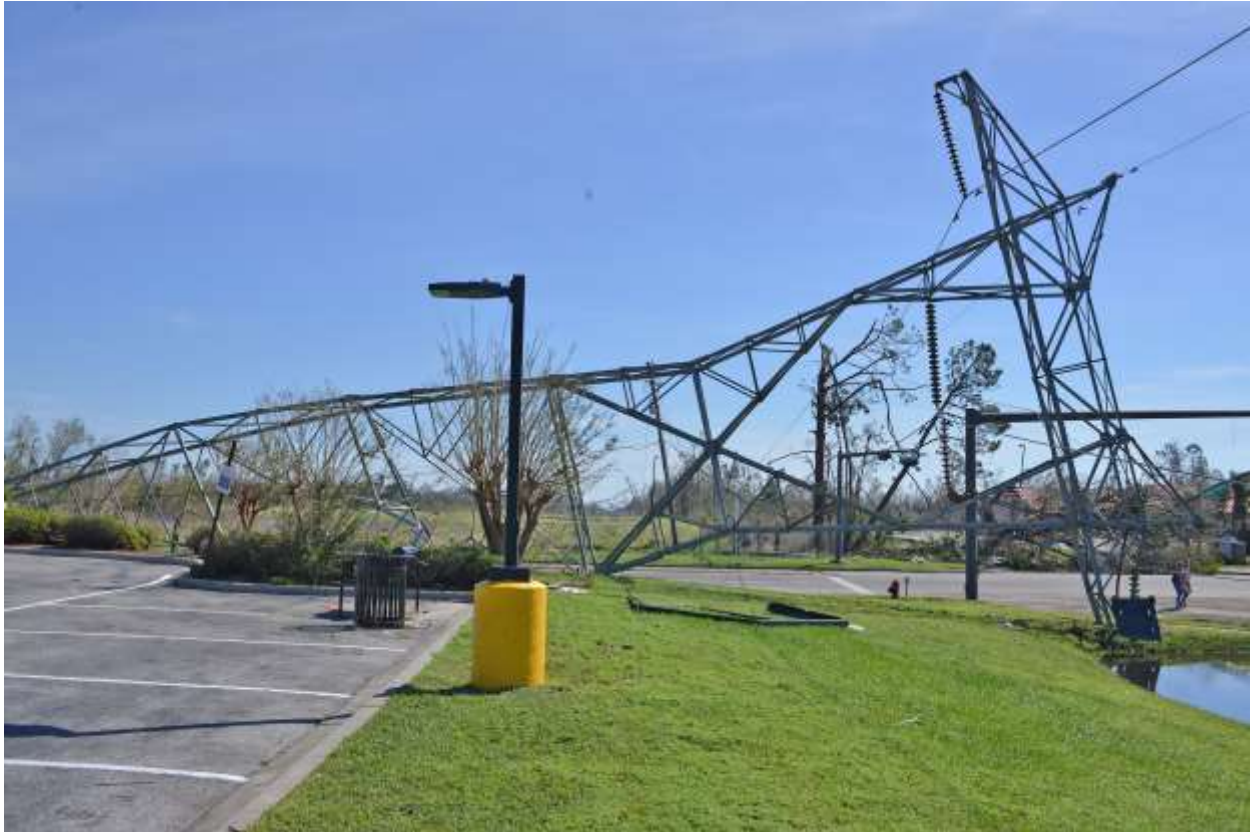
FIGURE 6 – STEEL LATTICE TOWER FAILURE
