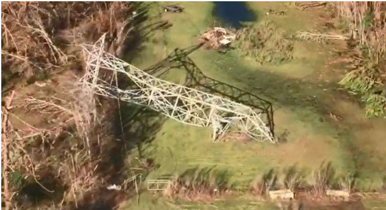
FIGURE 7 – STEEL LATTICE TOWER FAILURE
