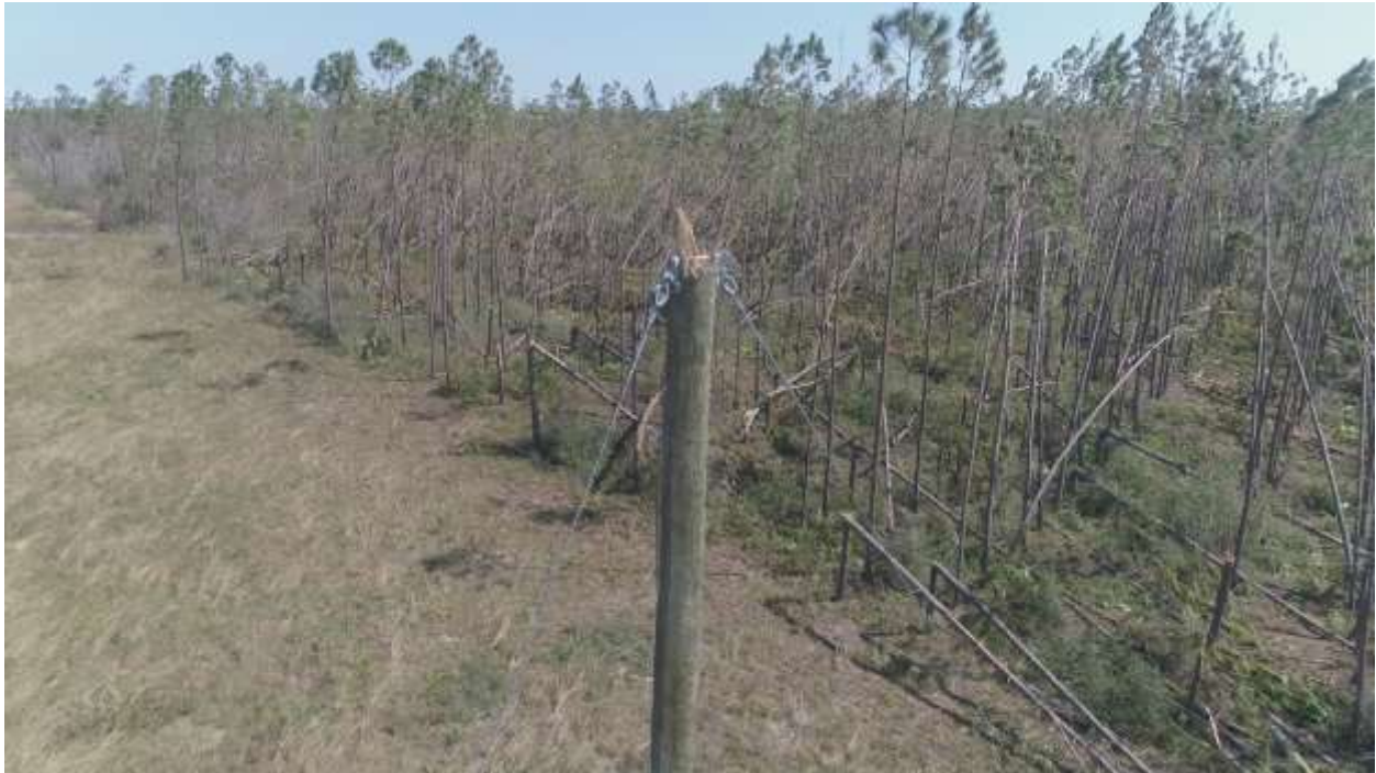
FIGURE 4 – WOOD POLE FAILURE AT STORM GUYS
