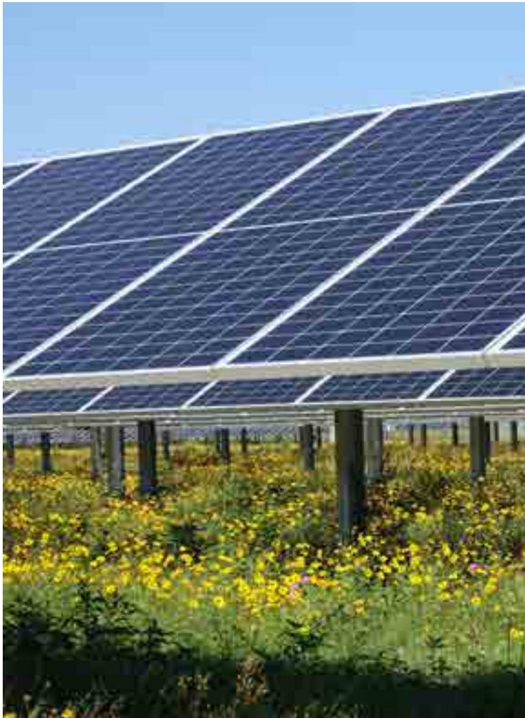
Wildflowers bloom at the FPL Echo River Solar Energy Center, Suwannee County
