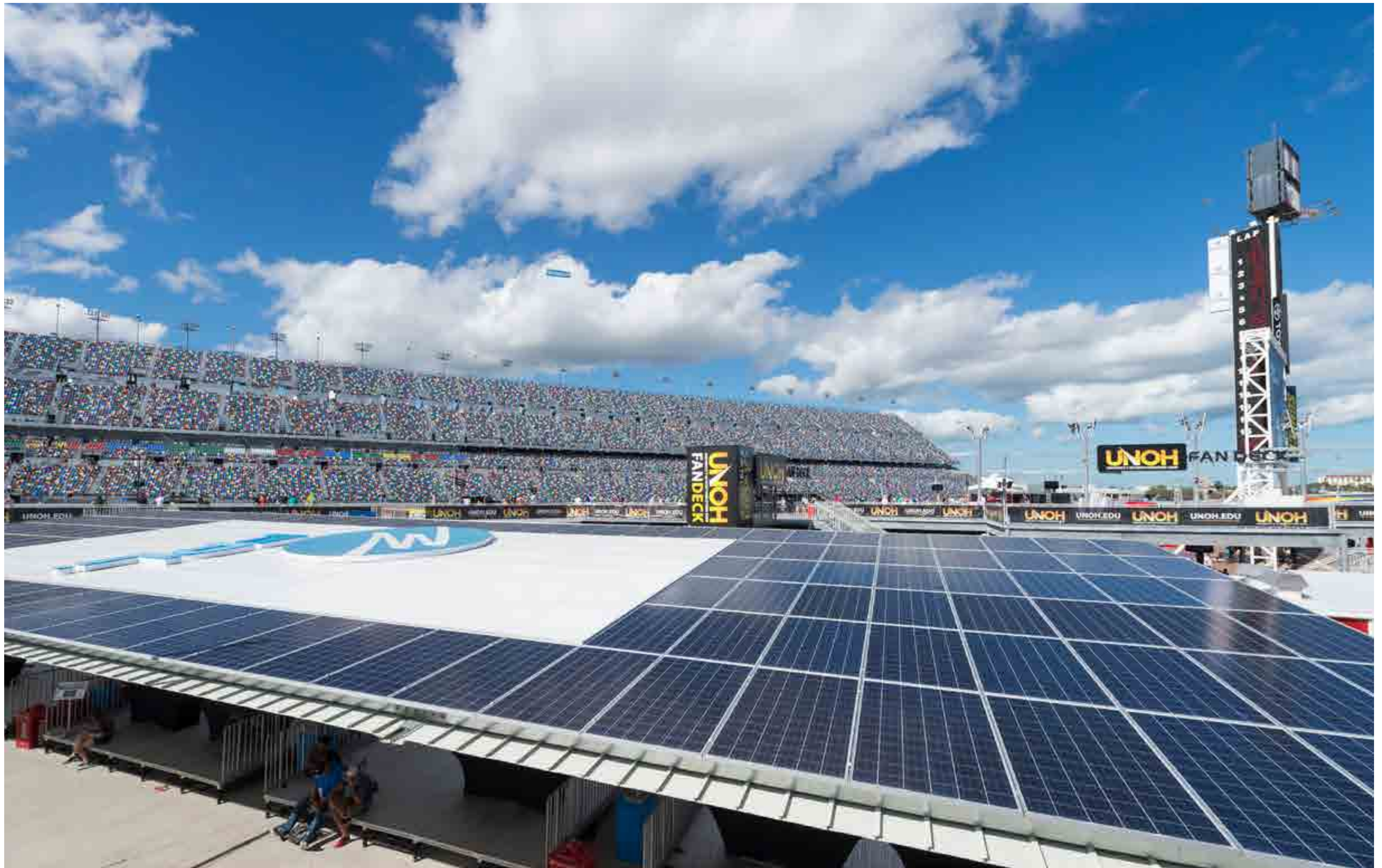
FPL Solar Circuit at Daytona International Speedway, Volusia County
