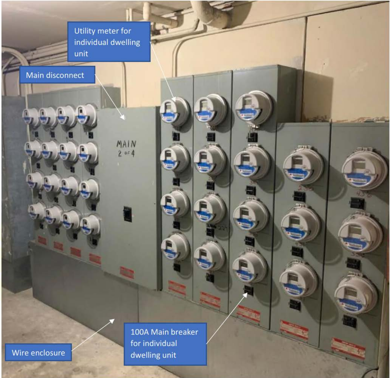
Photo 1: Meter Bank containing 24 meters
