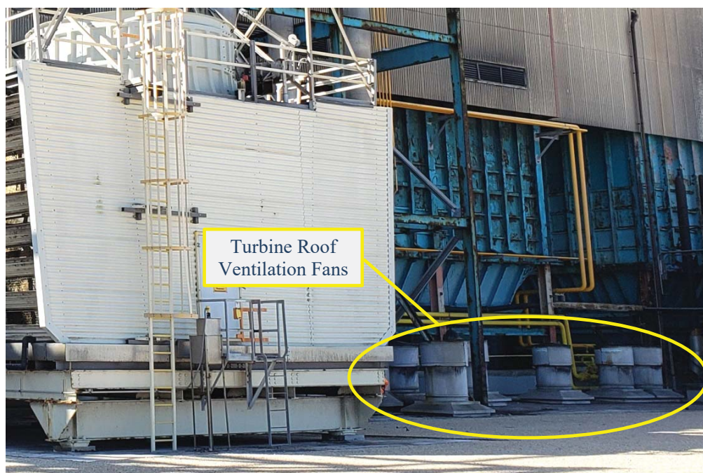
Figure 7 – Turbine Building Ventilation Fans
