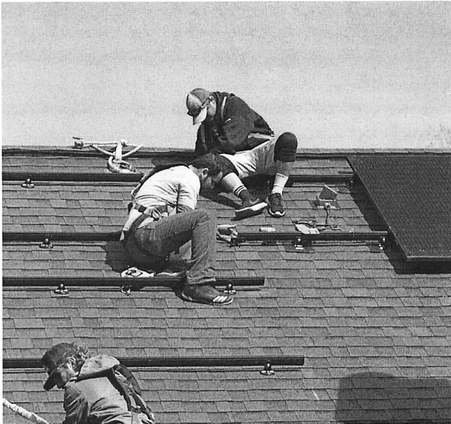
Sun Farm Energy workers on Feb. 8 install solar panels on a home in Escambia County.
