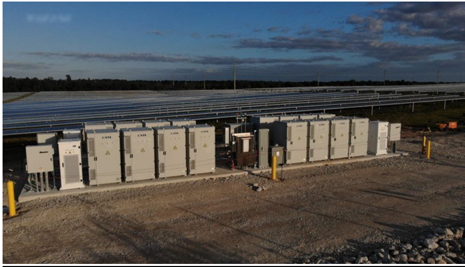
FIGURE 3.9 Lake Placid Battery Energy Storage System
