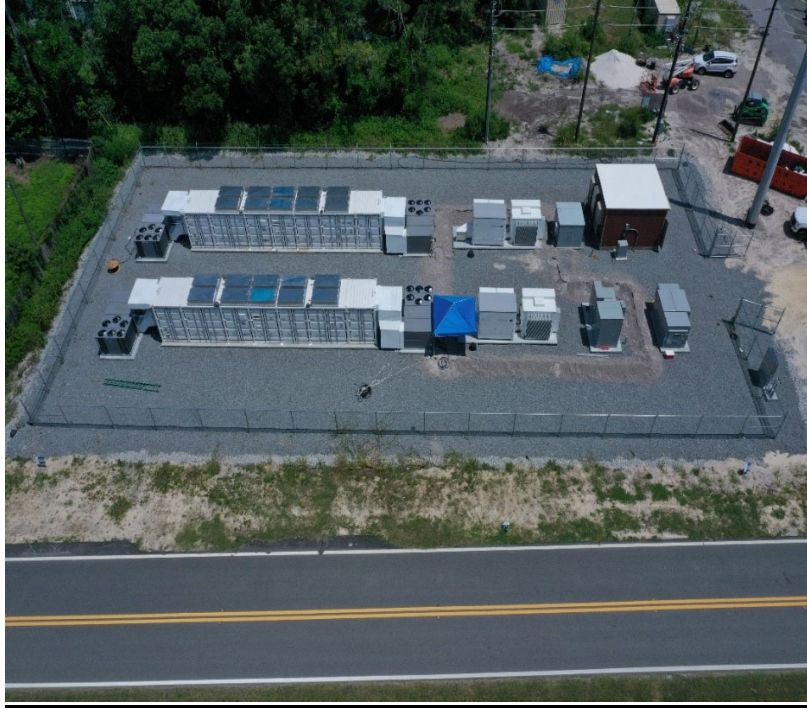
FIGURE 3.7 Jennings Battery Energy Storage System
