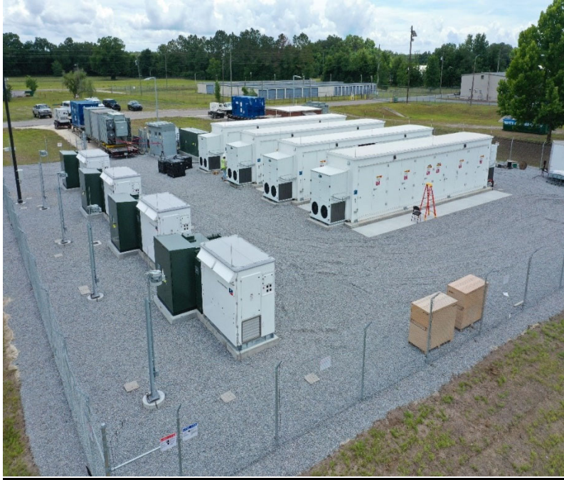
FIGURE 3.5 Trenton Battery Energy Storage System
