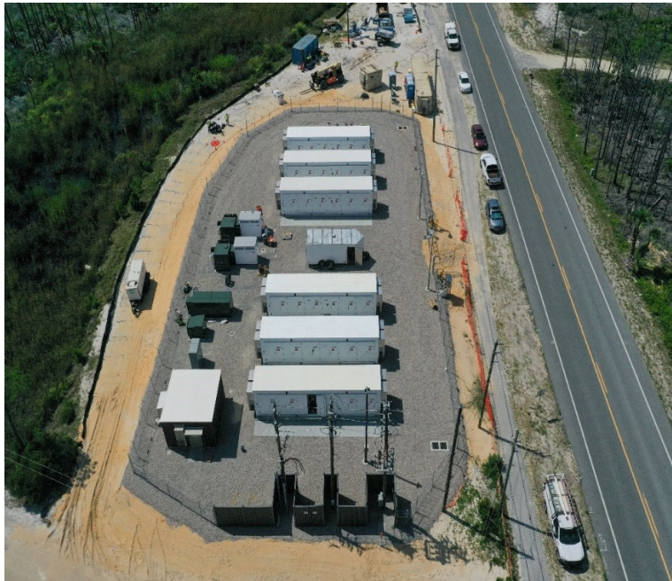
FIGURE 3.6 Cape San Blas Battery Energy Storage System
