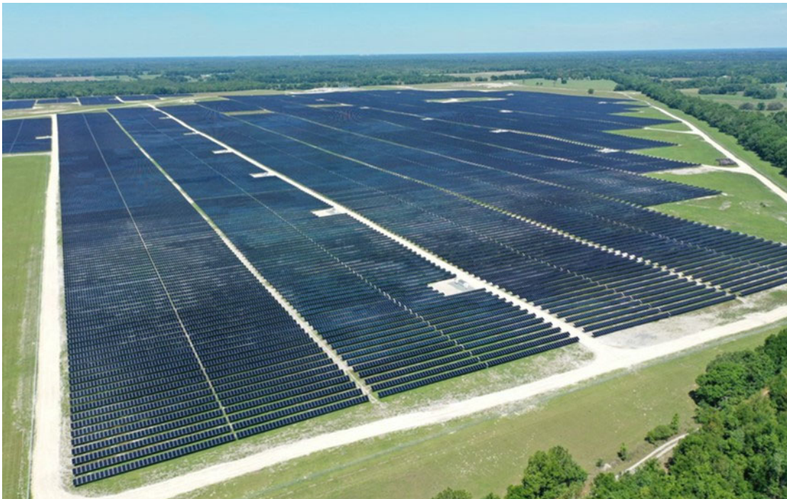
FIGURE 3.2 Santa Fe Solar Power Plant
