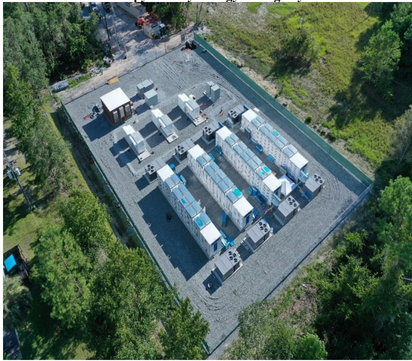
FIGURE 3.8 Micanopy Battery Energy Storage System
