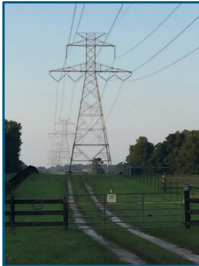
Figure 2: Double Circuit Tower
