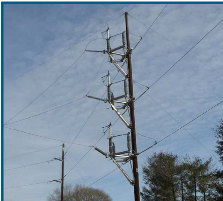
Figure 3: DEF Manually Operated Switch
