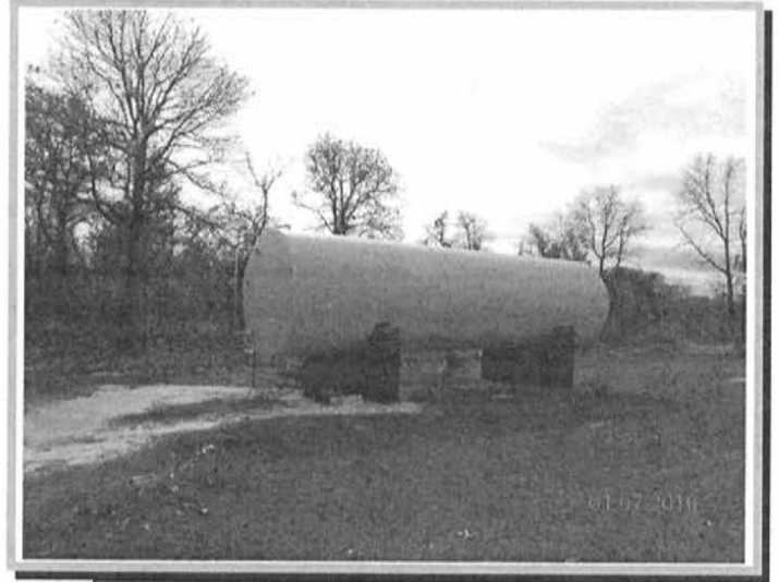
10,000 Gallon Ground Storage Tank at Plant #1
