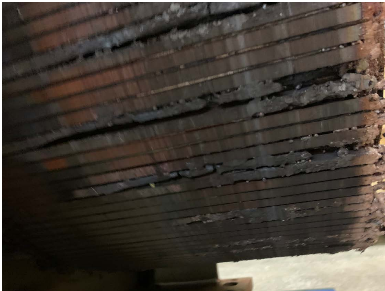
Fig. 6 PMG Stator Core – Coil Melt in Slots
