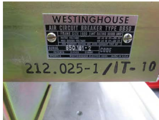
As Received Right Side of Breaker Platform
