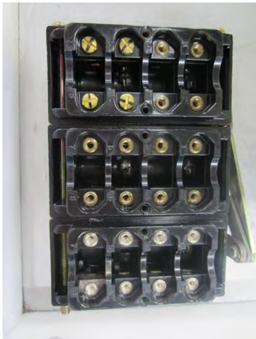
Front of Auxiliary Switches
