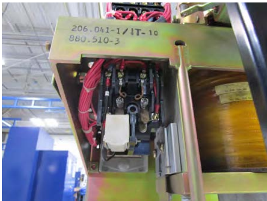
Control Relay with Front Cover Removed
