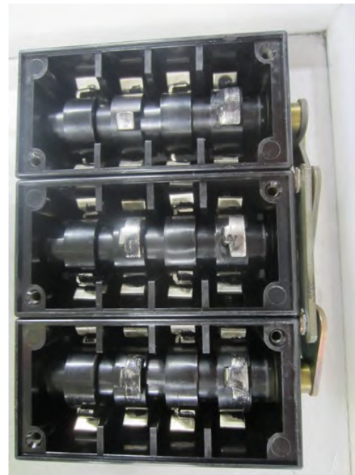
Rear of Auxiliary Switches
