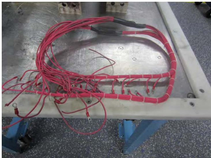
Breaker Wiring Harness
