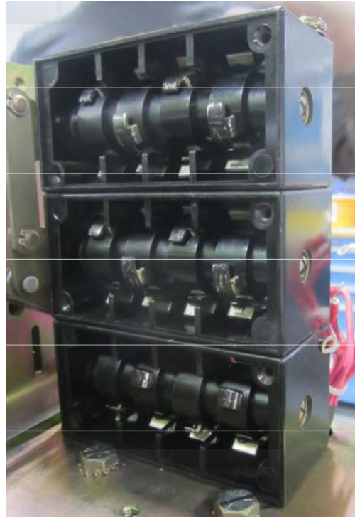
Rear of Auxiliary Switches
