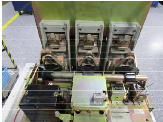
Breaker Open, With Arc Chutes Removed
