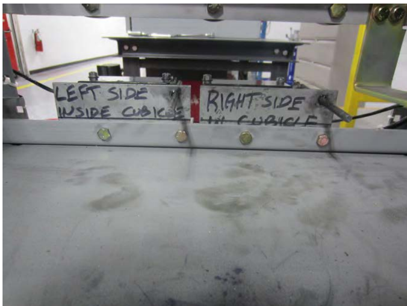
Left-Side Switch and Right-Side Switch Installed in Test Cell
