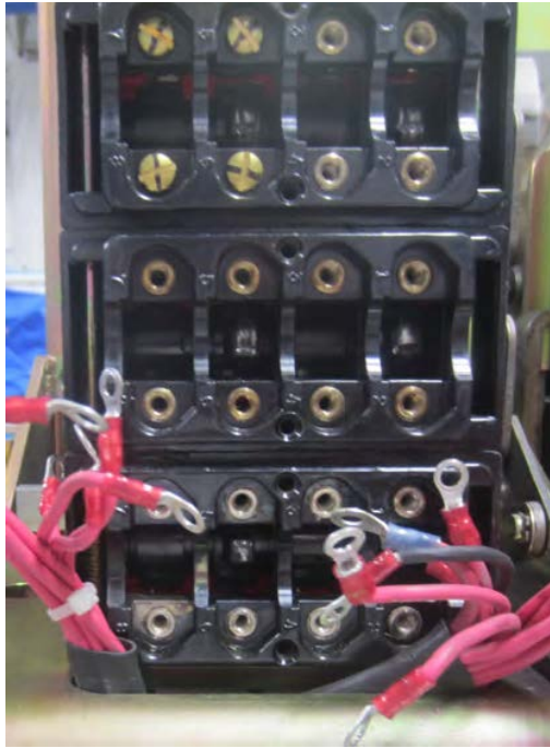
Front of Auxiliary Switches
