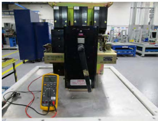
Breaker Closed, Switch Contact Open
