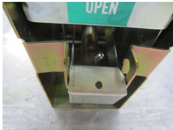
Bent Breaker Lock-Out Tabs
