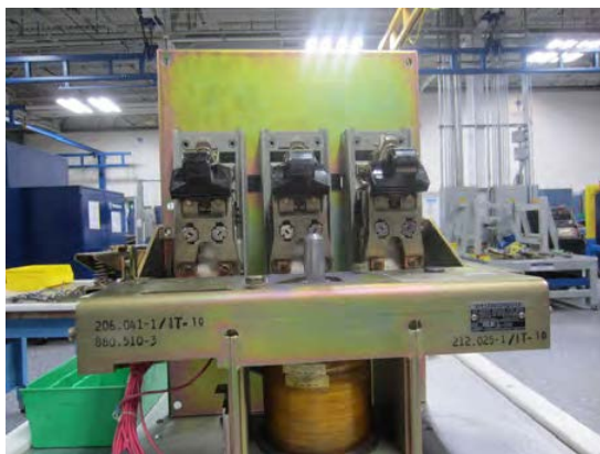
Breaker with the Operating Mechanism Removed
