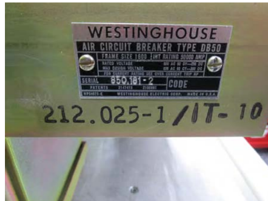
As Received Right Side of Breaker Platform
