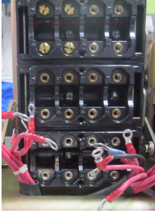
Front of Auxiliary Switches
