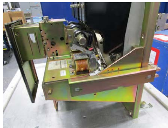
As Received Right Side of Breaker
