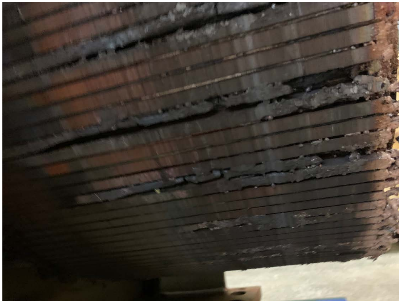
Fig. 6 PMG Stator Core – Coil Melt in Slots
