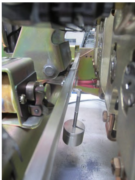
Additional Weight Added to the Operating Mechanism Trip Bar
