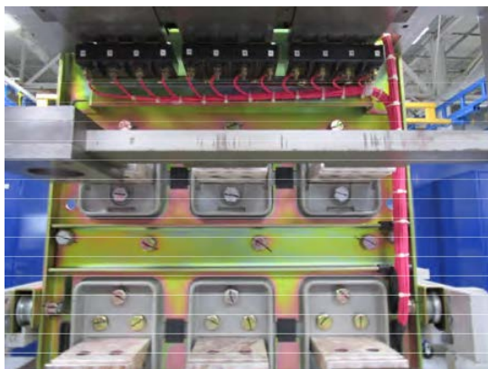
Breaker Stud Alignment
