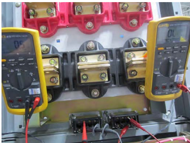
Switch Monitoring Shows a Change of State
