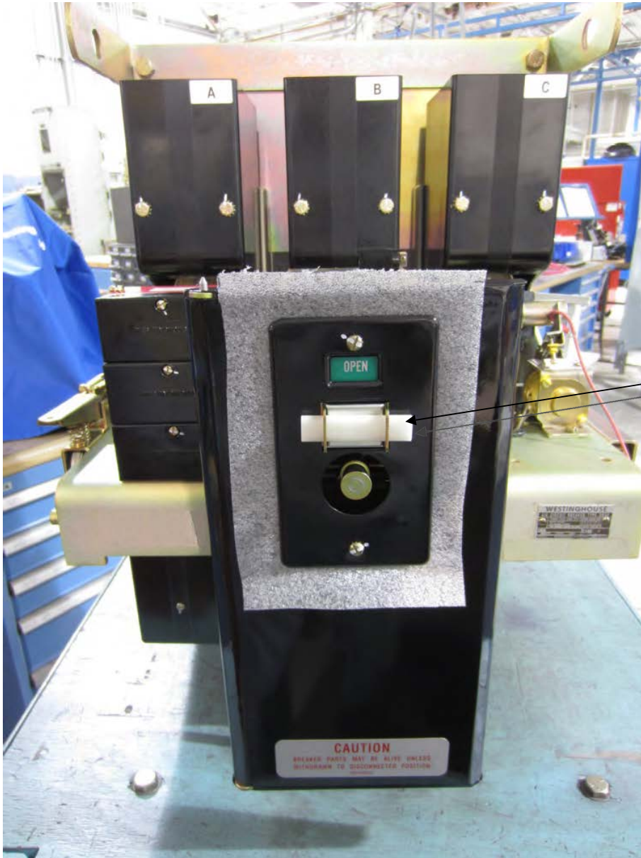
Refurbished DB-50 Breaker with Operating Mechanism Lock-Out Bar
