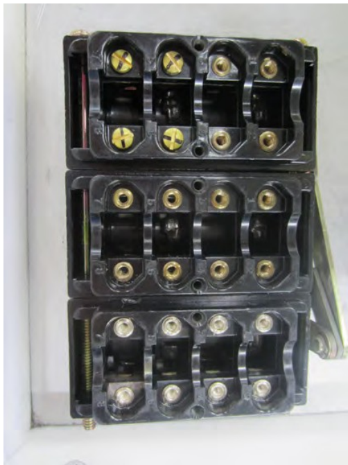
Front of Auxiliary Switches
