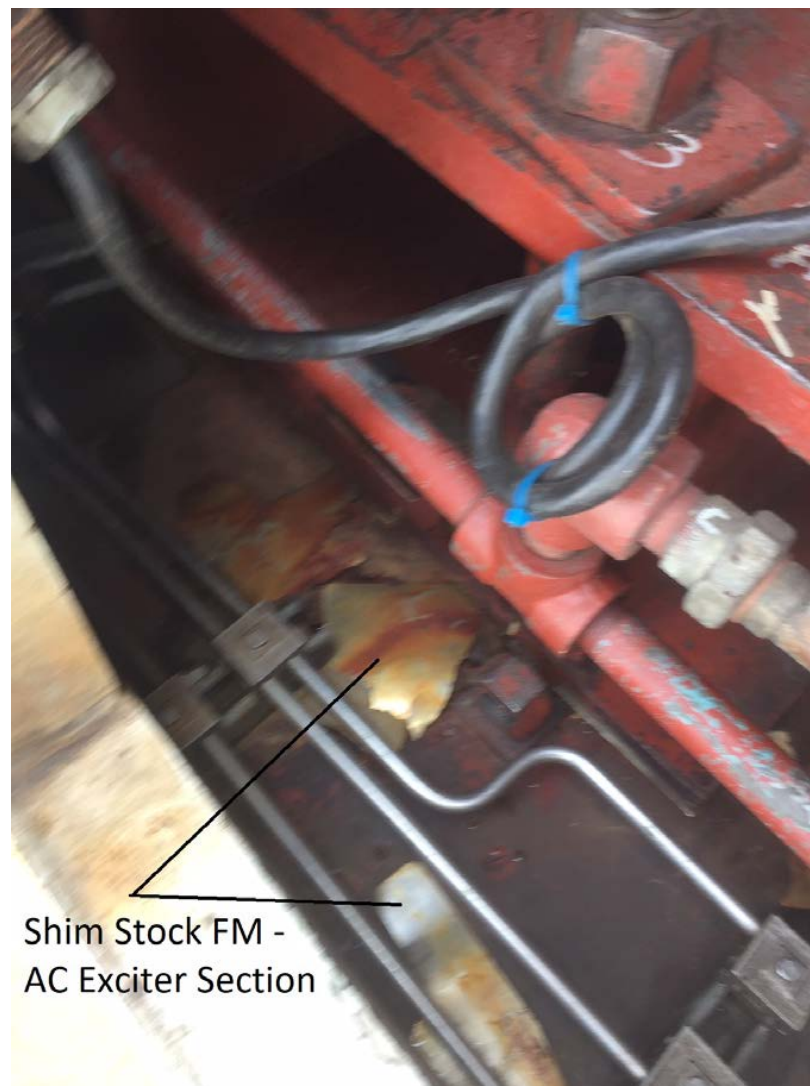
Fig. 11 Foreign Material (Shims) Found in AC Exciter Section
