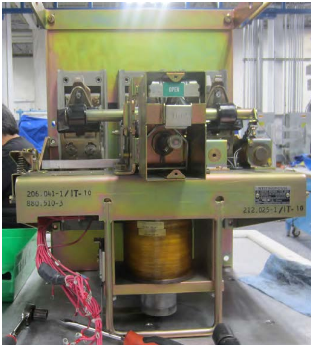
Breaker with the Auxiliary Switches and Control Relay Removed
