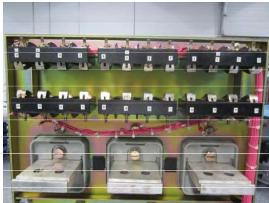
Secondary Contact Assembly on Breaker
