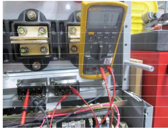
Left-Side Switch Monitoring (NC)
