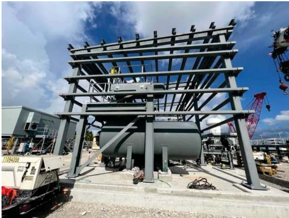
Glycol water heater tank on center. Enclosure on the left is the Power Distribution center.
