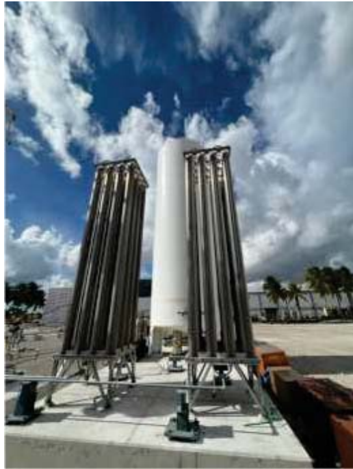
Nitrogen Tank and Vaporizers
