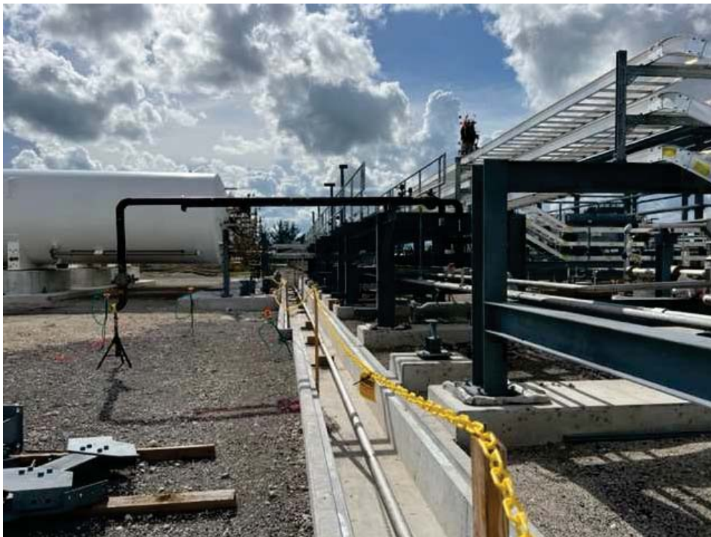
North side of LNG tanks, pipe rack and cable tray. Spill trench on center.
