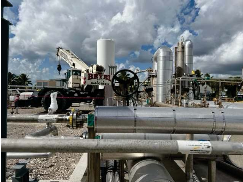
Truck unloading pump skid and white Nitrogen tank in the background
