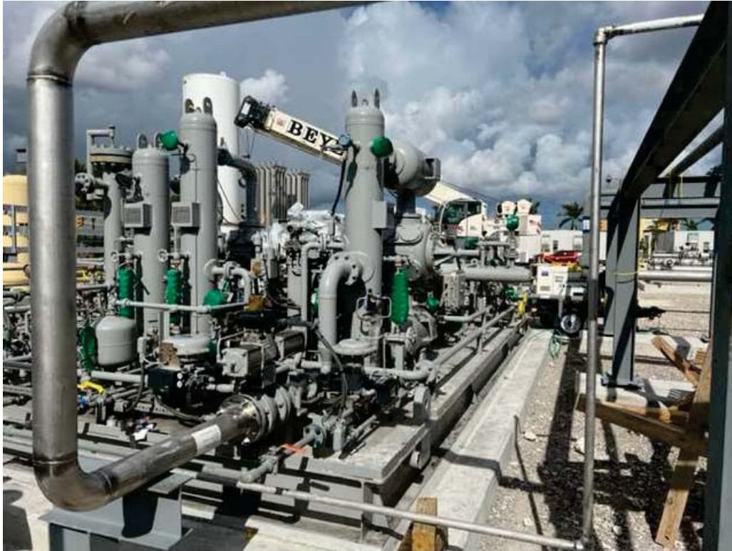
Boil-Off Gas Compressor
