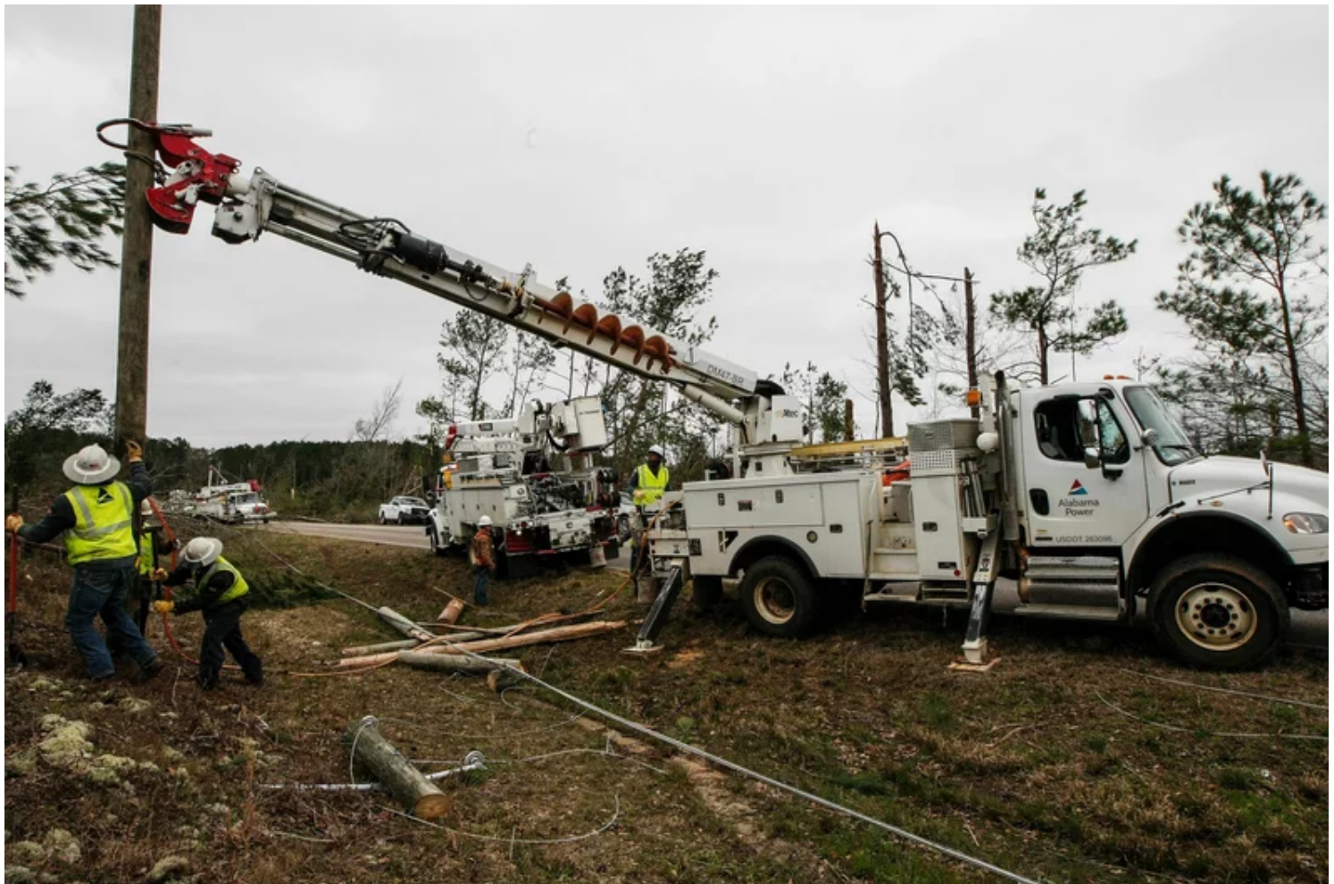
Alabama Power begins putting up poles to get power restored in Bearegard, Ala., after a tornado in 2019. The power company was a client of Matrix.
