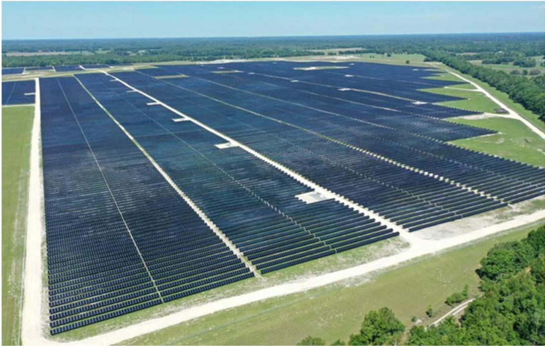
FIGURE 3.2 Sandy Creek Solar Power Plant
