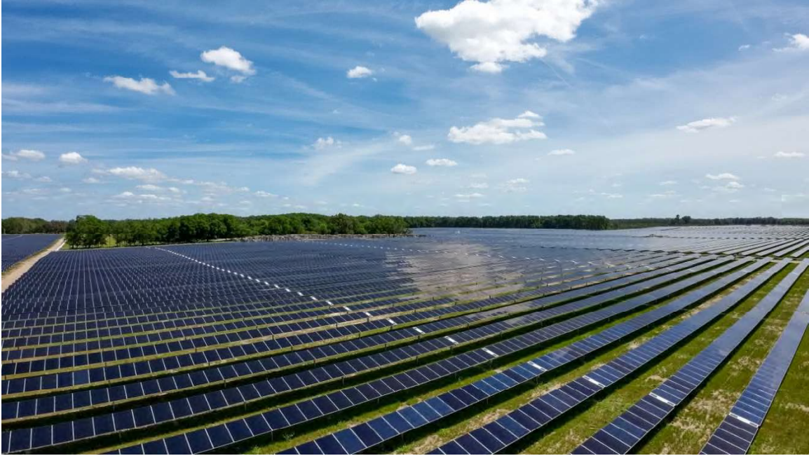
FIGURE 3.4 High Springs Solar Power Plant
