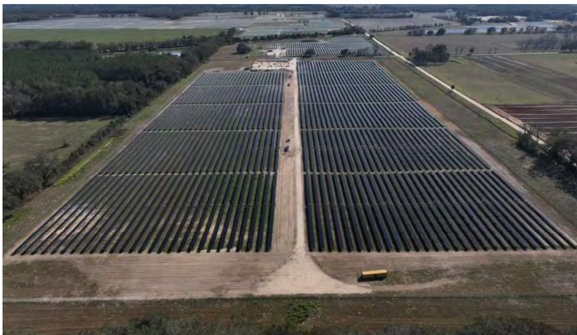
FIGURE 3.3 Hardeetown Solar Power Plant
