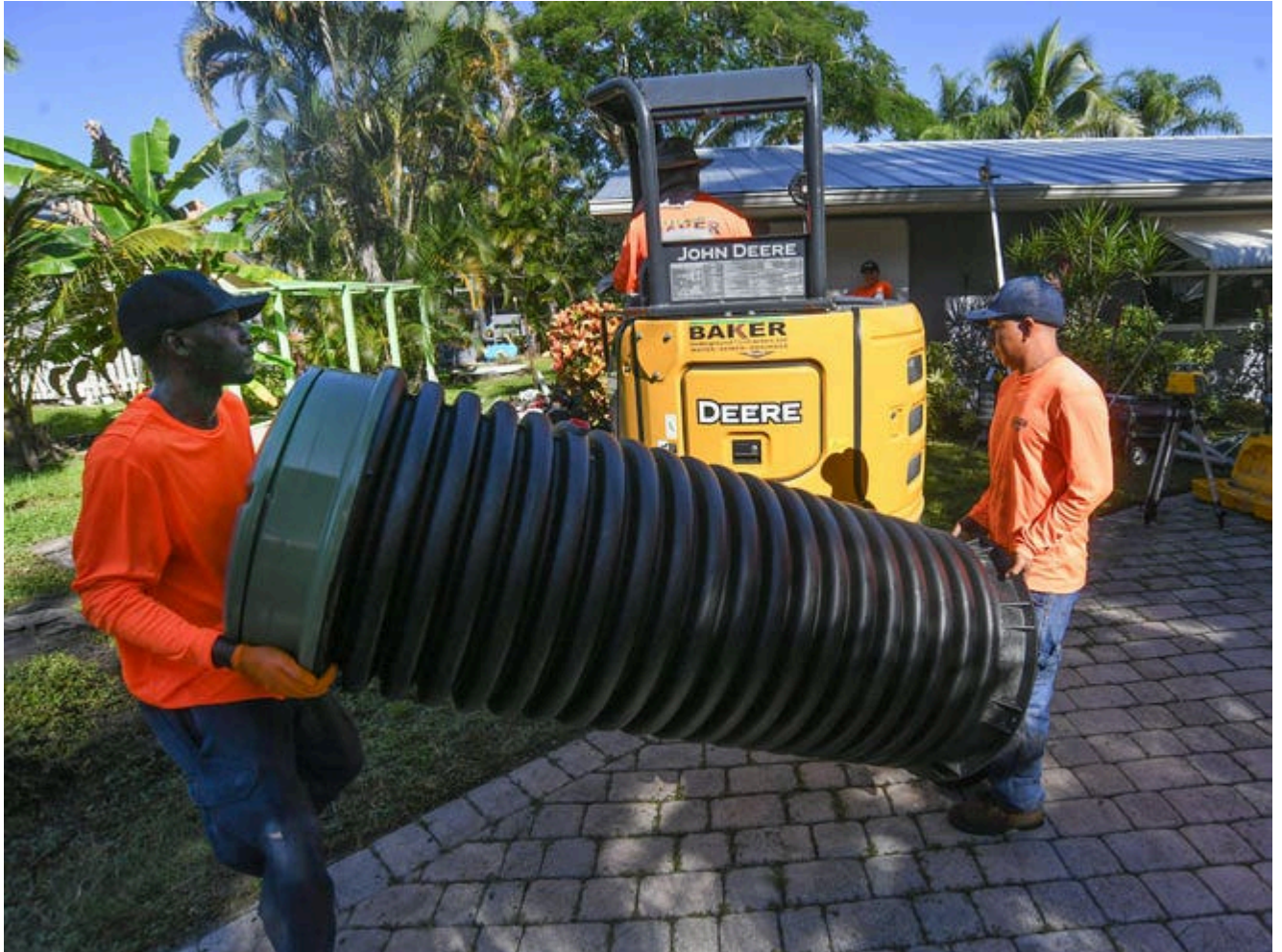
The crew of Baker Underground Contractors works to install a new E1 grinder system residential station replacing an older septic system as part of Martin County's septic-to-sewer program at a home on Southwest St. Lucie Street on Friday, Oct. 20, 2023, in Stuart.
