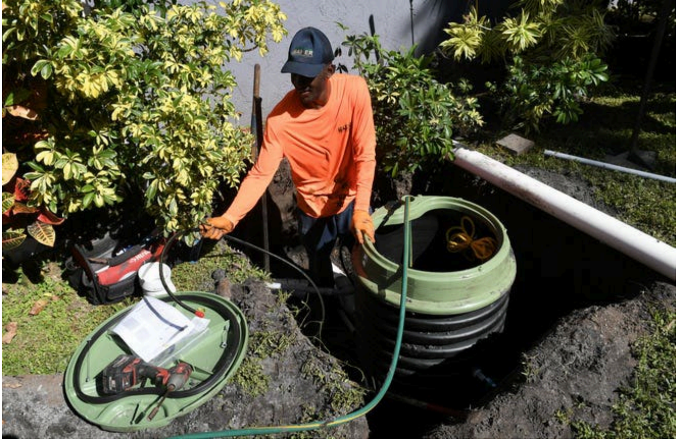
The crew of Baker Underground Contractors works to install a new E1 grinder system residential station replacing an older septic system as part of Martin County's septic-to-sewer program at a home on Southwest St. Lucie Street on Friday, Oct. 20, 2023, in Stuart.
