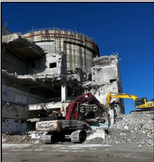
Control Complex Demo
