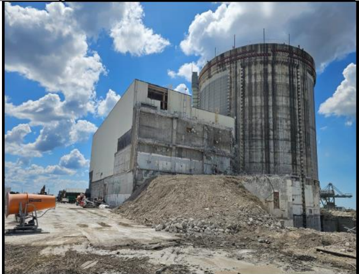
Control Complex Demo
