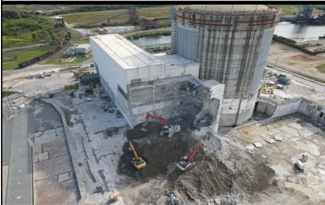
Control Complex Demo
