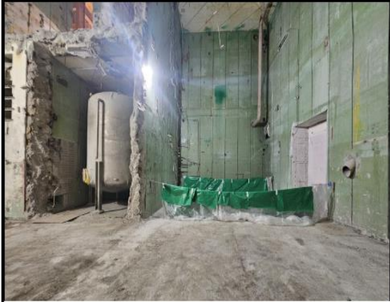
AB Spent Resin Tank
