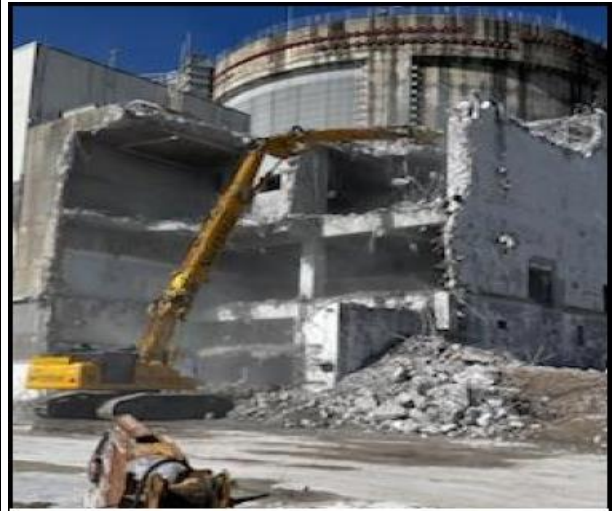
Control Complex Demo
