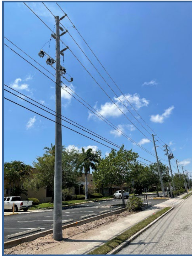
Figure 2: Hardened distribution feeder including structures that have been strengthened to the NESC 250C standard and increased BIL from hardware and spacing upgrades.
