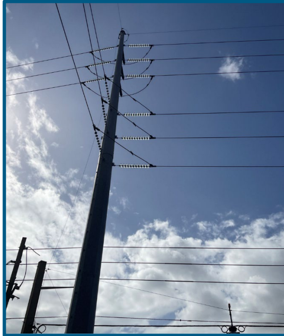
Figure 6: Failed static due to extreme weather event.
