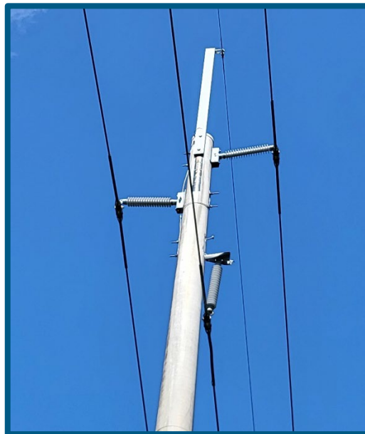
Figure 7: Failed porcelain insulator due to extreme weather event.
