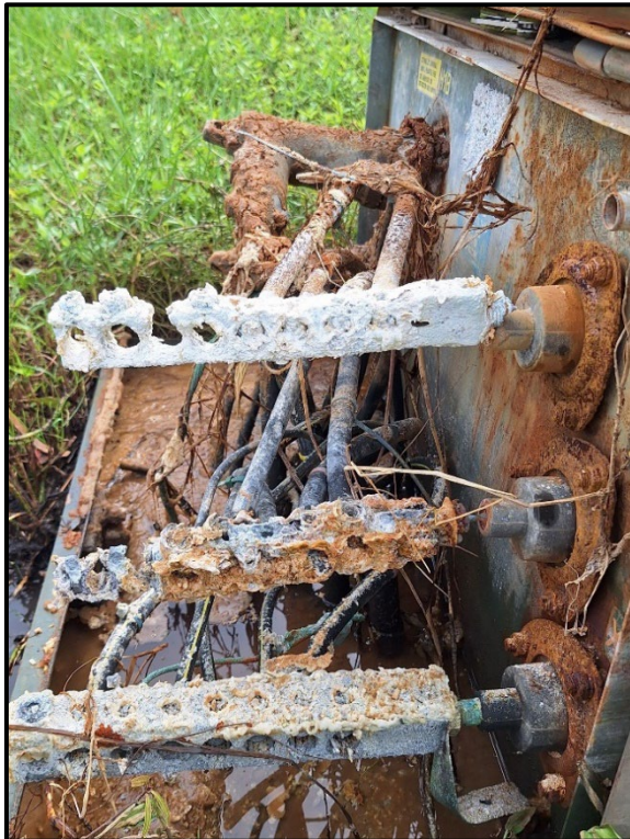
Figure 1: Underground construction with severe corrosion and electrolysis due to storm surge during Hurricane Helene
