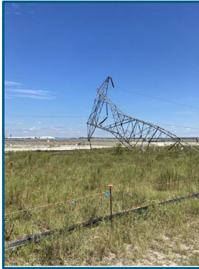
Figure 4: Lattice Tower impacted by Hurricane Idalia
