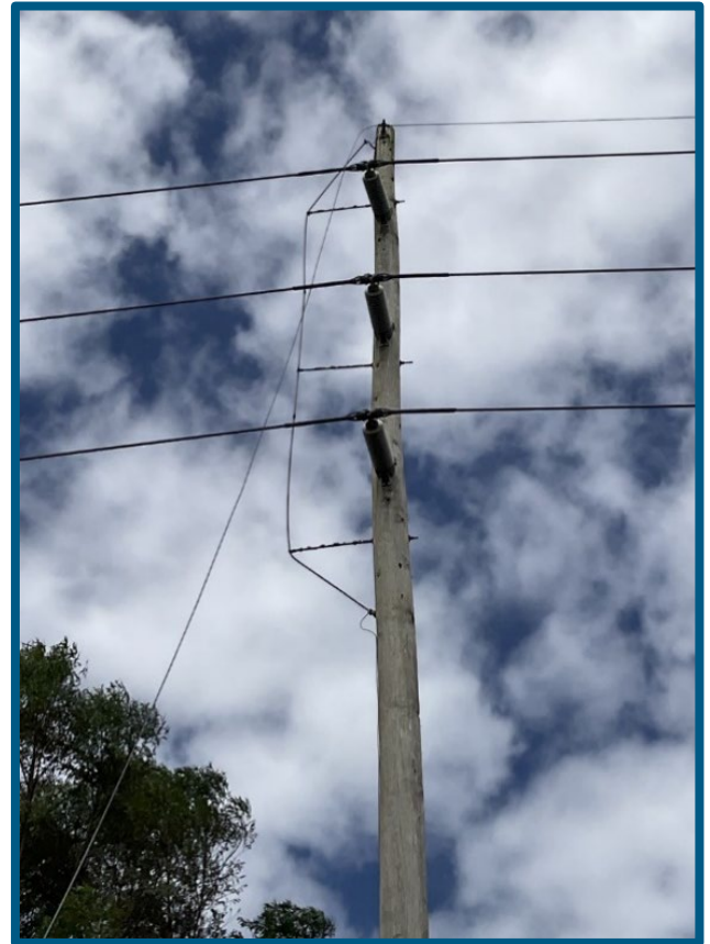
Figure 2: Broken Static due to extreme weather event.
