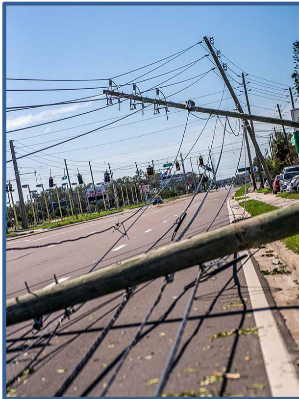
Figure 1: Distribution feeder poles broken by straight line winds from Category 3 hurricane.
