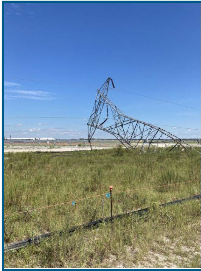
Figure 4: Lattice Tower impacted by Hurricane Idalia
