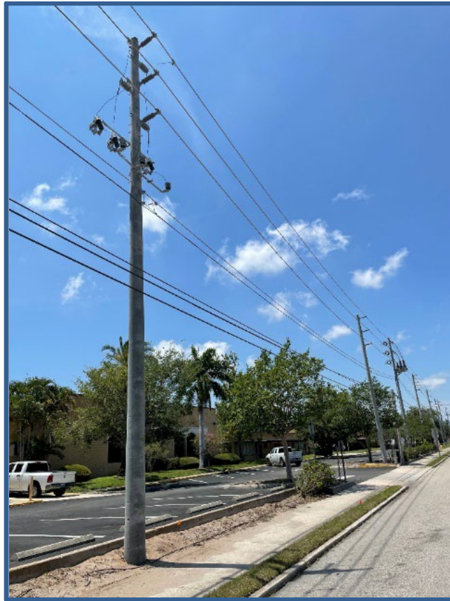
Figure 2: Hardened distribution feeder including structures that have been strengthened to the NESC 250C standard and increased BIL from hardware and spacing upgrades.
