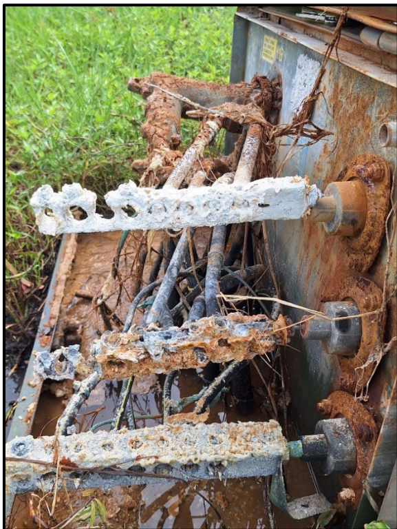
Figure 1: Underground construction with severe corrosion and electrolysis due to storm surge during Hurricane Helene
