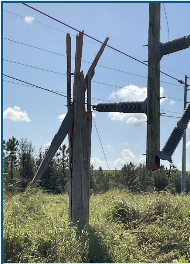
Figure 1: Broken Pole due to extreme weather event.
