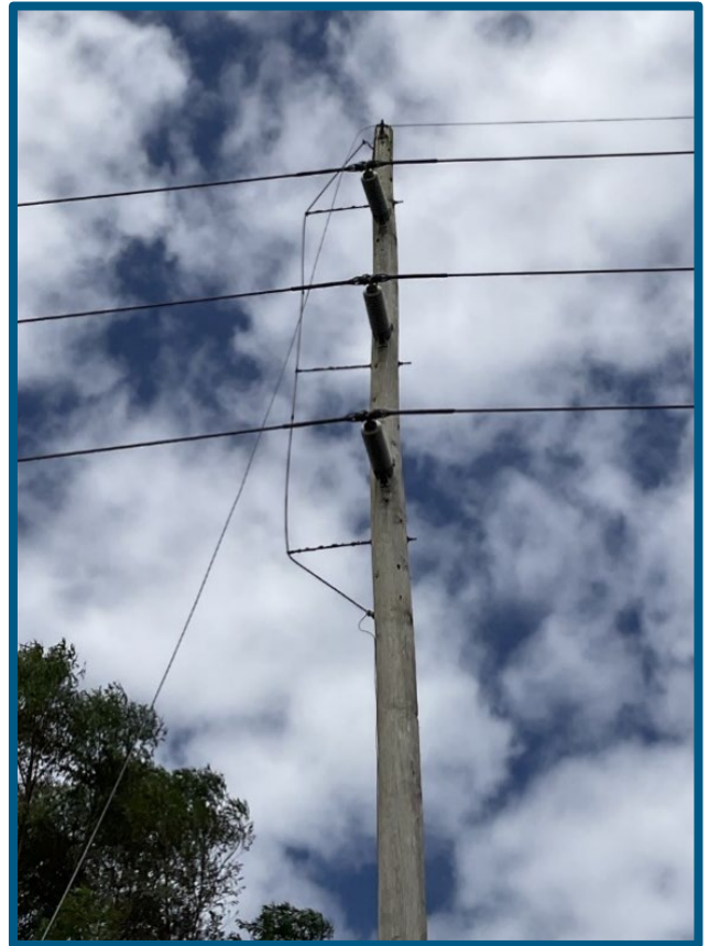
Figure 2: Broken Static due to extreme weather event.
