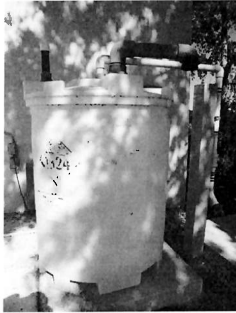
Photo 2: View of the sulfuric acid.
