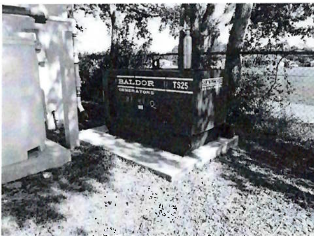
Photo 9: On site manual generator.
