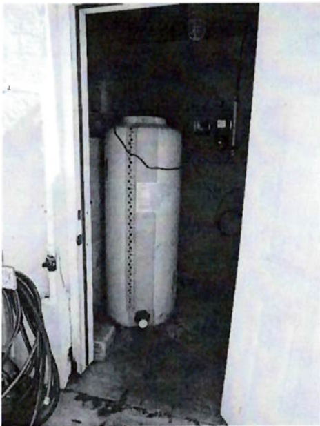
Photo 5: View of chlorine.
