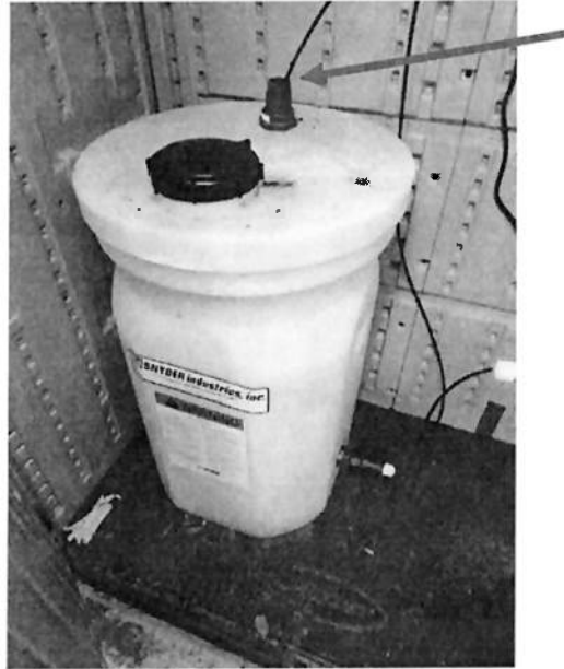
Photo 4: View of ammonia. Not secured.
