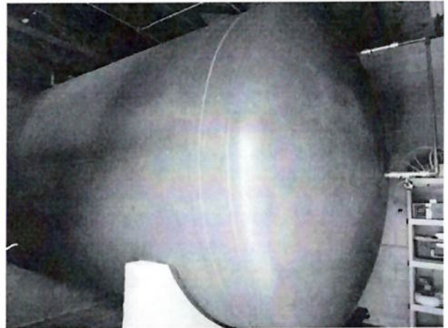
Photo 6: View of hydro-pneumatic tank.
