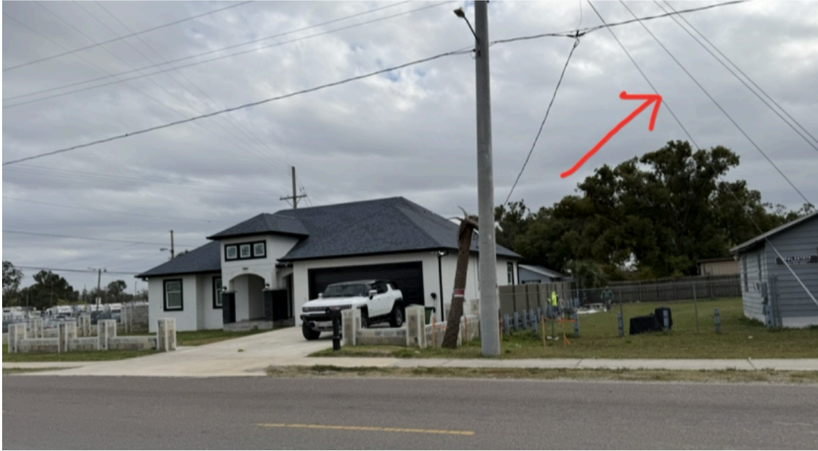
After Photograph – Relocated Pole and Guy Wire Placement (Shows facilities relocated in front of Petitioner’s front entrance)
