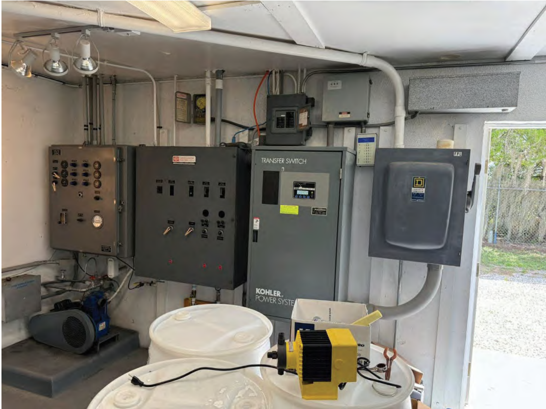
Photo # 34 – Well Control Panel, ATS, Electrical and Air compressor
