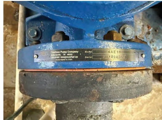
Photo # 30 – Pump No. 3
