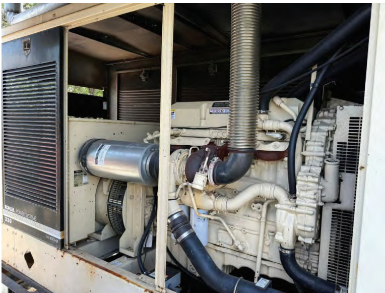
Photo # 55,56,57 – Emergency Generator
