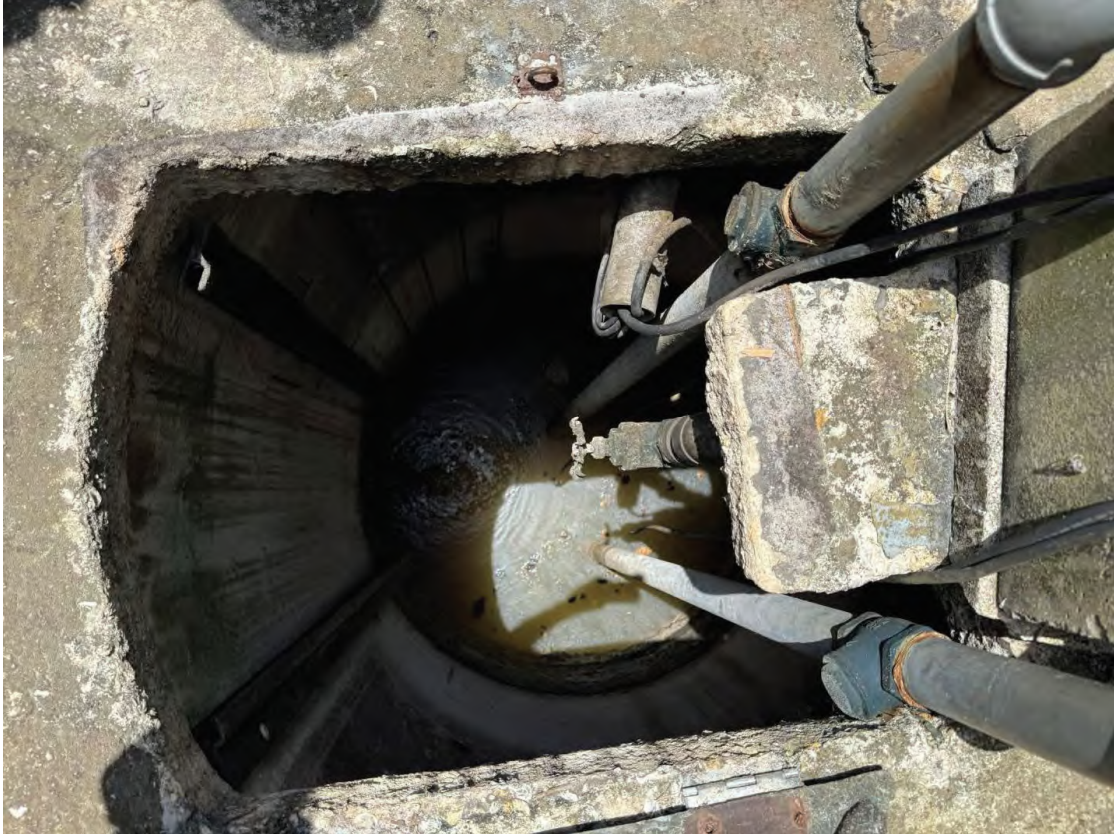
Photo # 70 – Lift Station No. 1 (Golf Course) Wetwell
