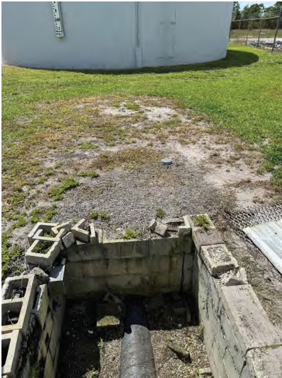
Photo #14 – Yard Vault North-East of GSR No.2
