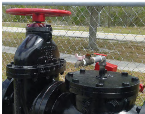
Photo 6: Well Head #3 Raw Water Tap
