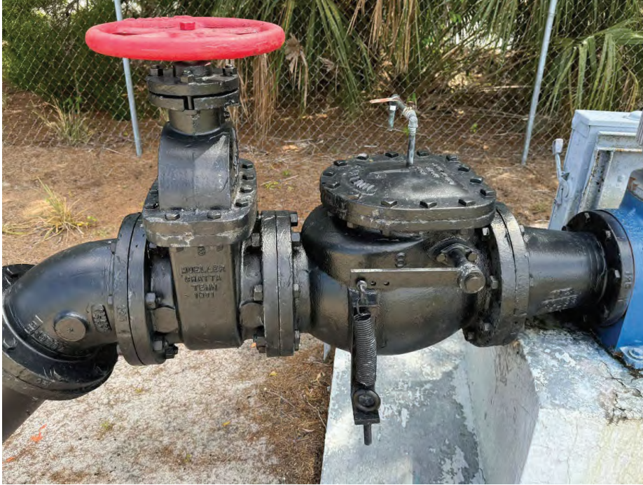
Photo #5 – Well No.1 – Effluent Piping
