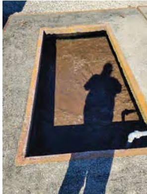
5. Aeration Basin (on)
