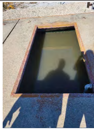
2. Aeration Basin (off)
