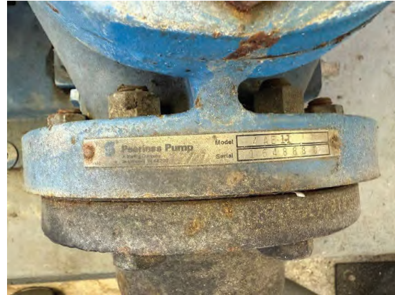
Photo # 28 – Pump No. 2
