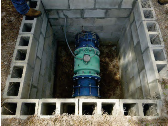
Photo 25: Finished Water Flow Meter
