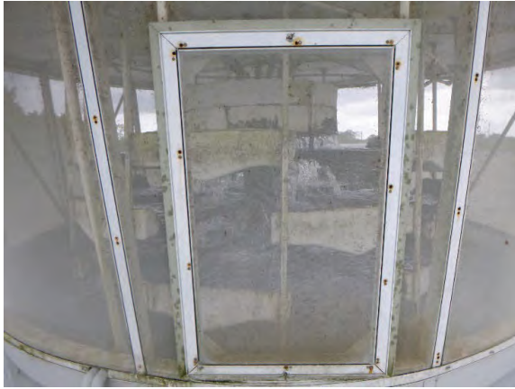
Photo 13: Ground Storage Tank #1 Aerator
