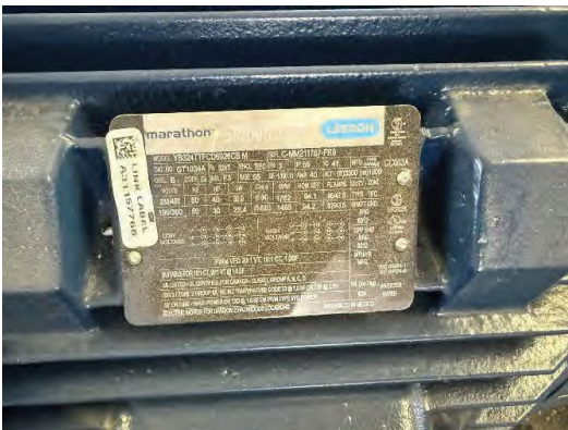
Photo # 25 – Pump No. 1 Motor
