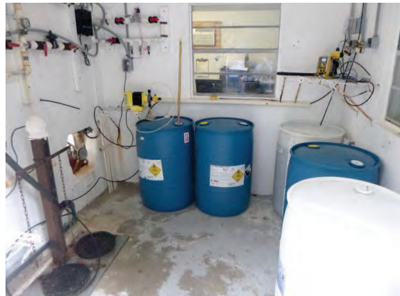
Photo 22: Hydrogen Peroxide Storage
