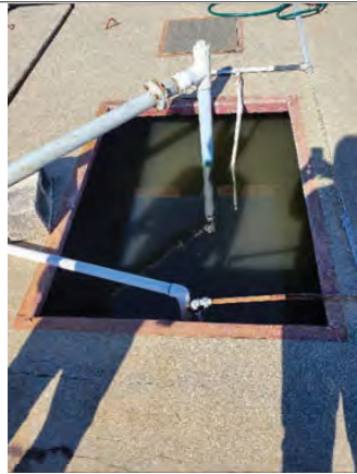
1. Aeration Basin (off)
