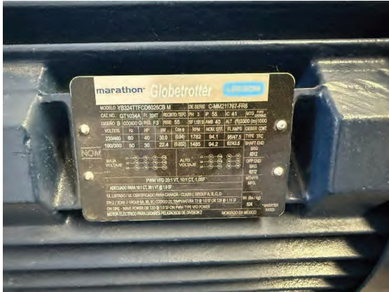
Photo # 27 – Pump No. 2 Motor
