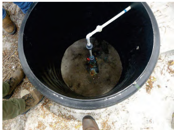
Photo 24: Chlorine Injection Site
