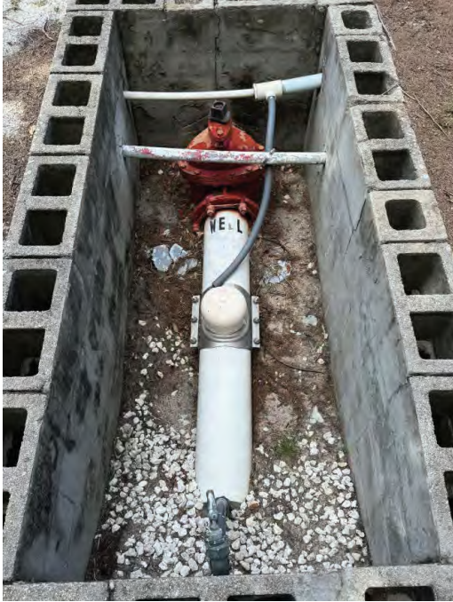
Photo #15 – Pressure Sensor Well No.1 Vault
