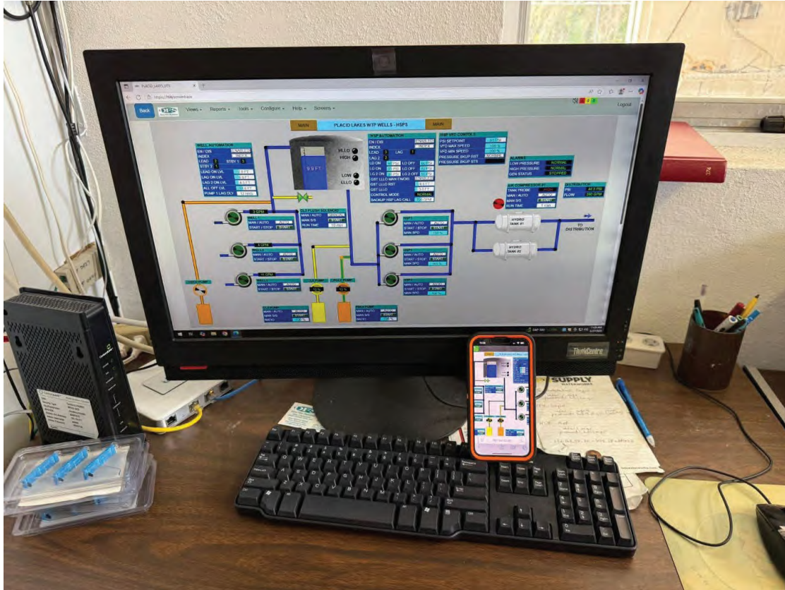
Photo # 37 – Dataflow SCADA
