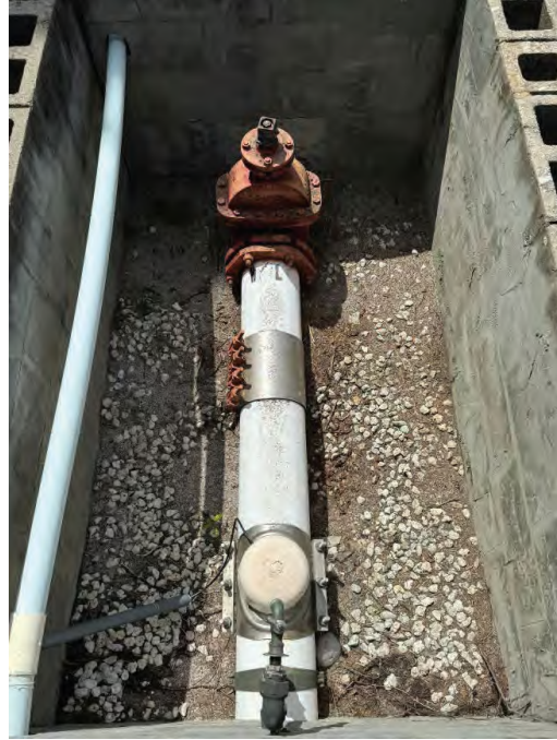
Photo #16 – Pressure Sensor Well No.2&3 Vault
