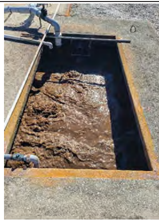
4. Aeration Basin (on)
