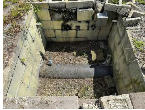
Photo #18 – Chlorine Injection Point No.2 Vault
