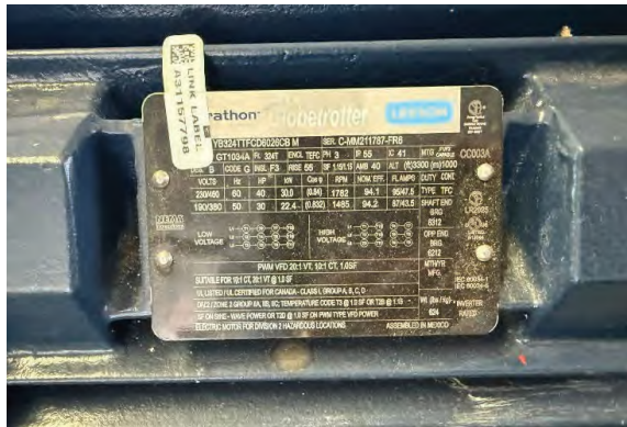
Photo # 29 – Pump No. 3 Motor
