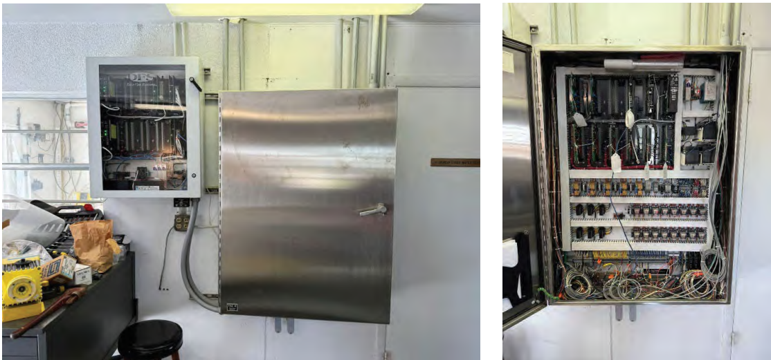
Photo # 35, 36 – Dataflow Instrumentation Panel
