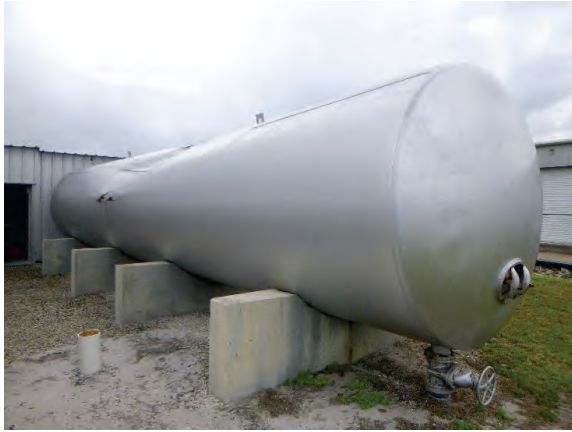
Photo 19: Hydro-Pneumatic Tank #3 (Imploded)
