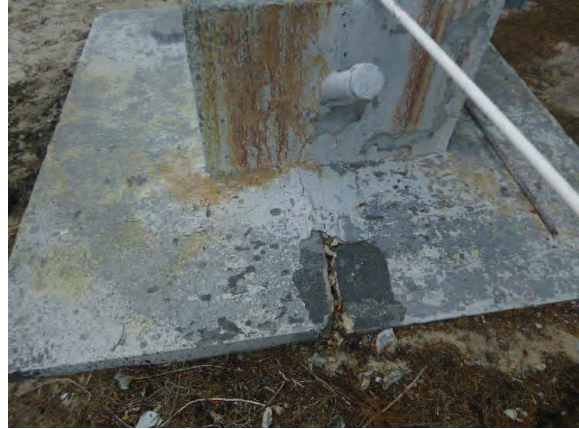
Photo 2: Well Head #1 Cracked Pad
