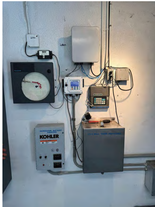
Photo # 33 – Electrical and Records
