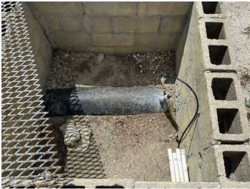
Photo #17 – Chlorine Injection Point No.1 Vault
