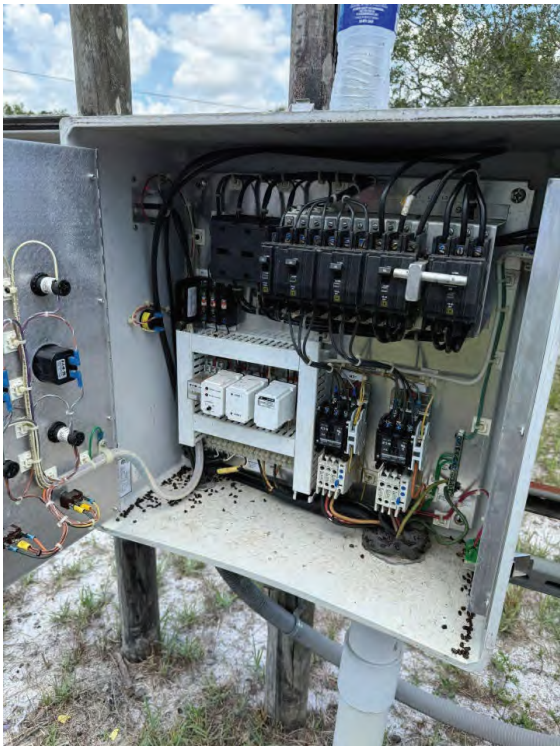
Photo # 72,73,74 – Lift Station No. 2 (Condos) Control Panel
