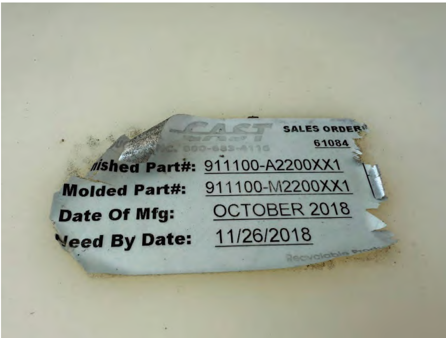
Photo # 46, 47, 48 – Chlorine Tank
