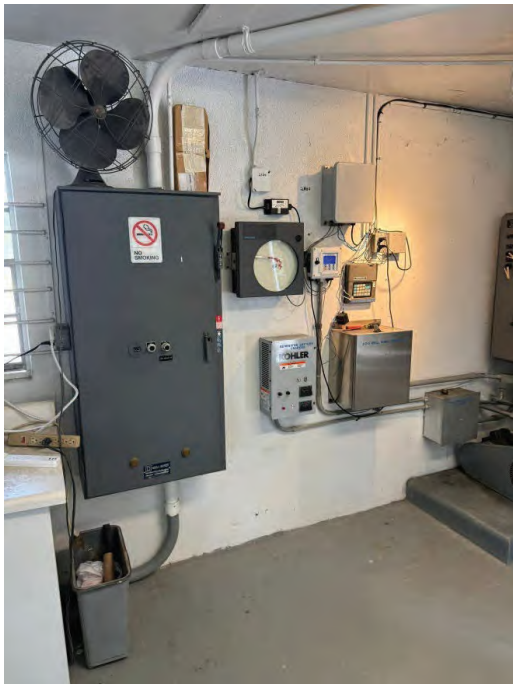
Photo # 32 – HSP Control Panel
