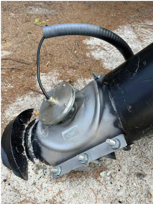
Photo #6 – Well No.1 – Effluent Flowmeter
