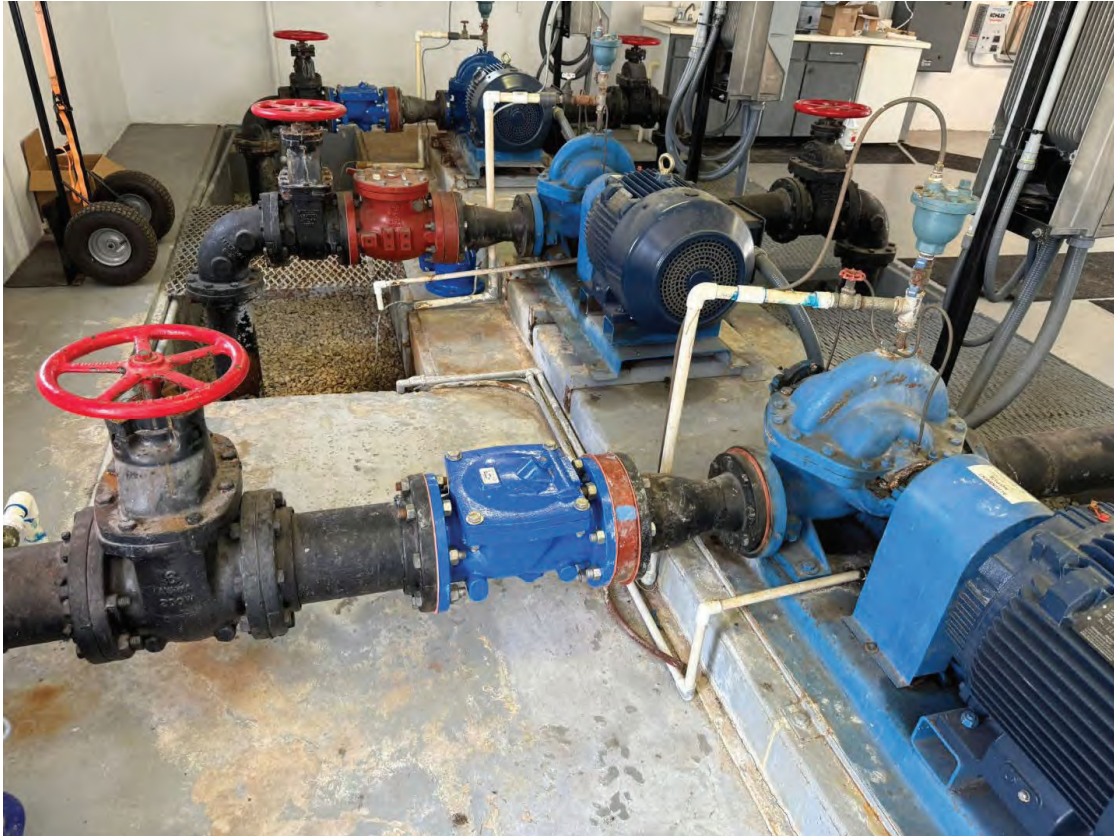
Photo # 24 – Pump Room
