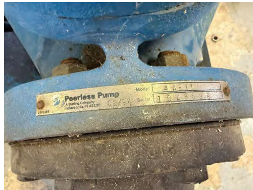
Photo # 26 – Pump No. 1
