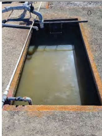
3. Aeration Basin (off)
