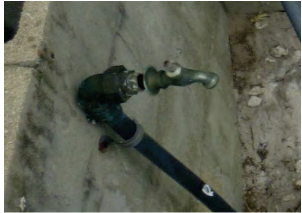
Photo 8: Well #2 Threaded Raw Water Sample Tap
