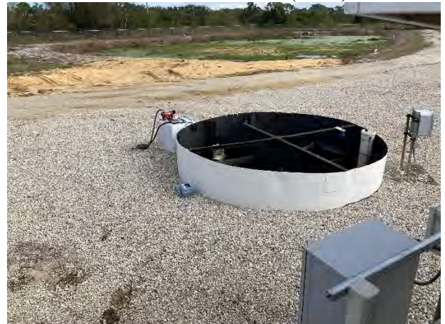
24. Chlorine Contact Chamber (CCC)
