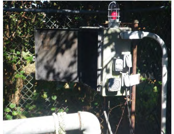
22 Shad Dr. electrical box
