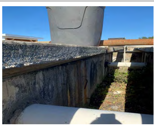
6. Trash can leaking onto ground
