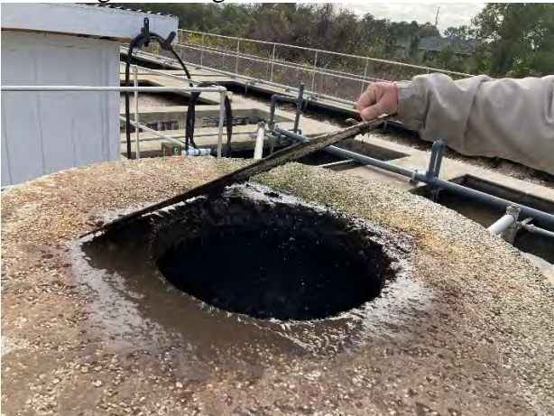
21. Sludge Holding Tank
