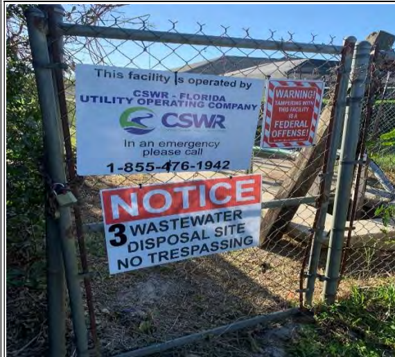
33. Signage on lift station
