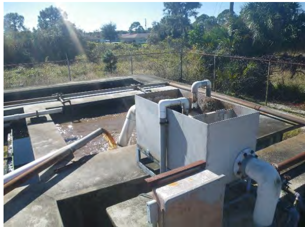
6 Surge tank to first aeration basin
