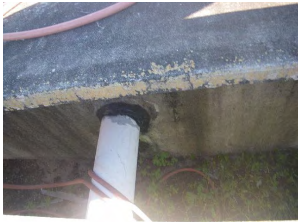
12 Leak around pipe connection
