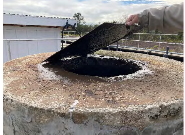
20. Sludge Holding Tank
