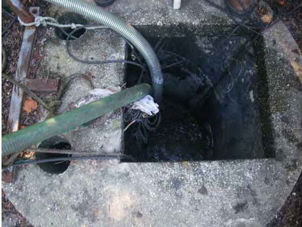
19 Clam Dr. lift station
