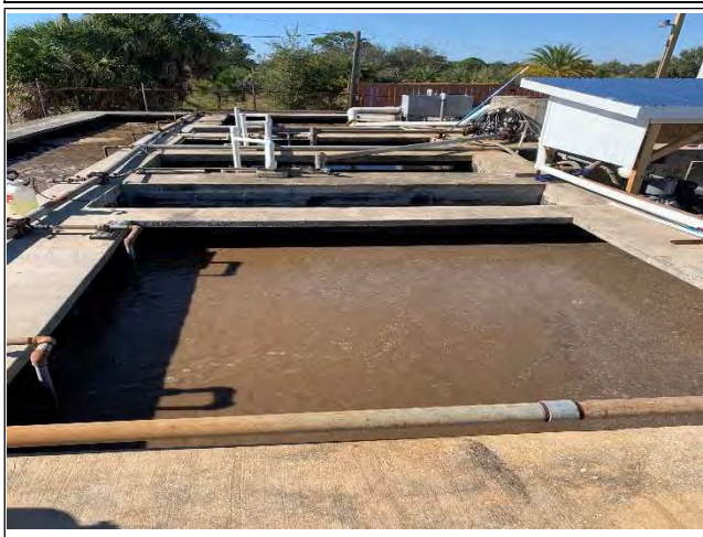
18. Aeration basin (anoxic)
