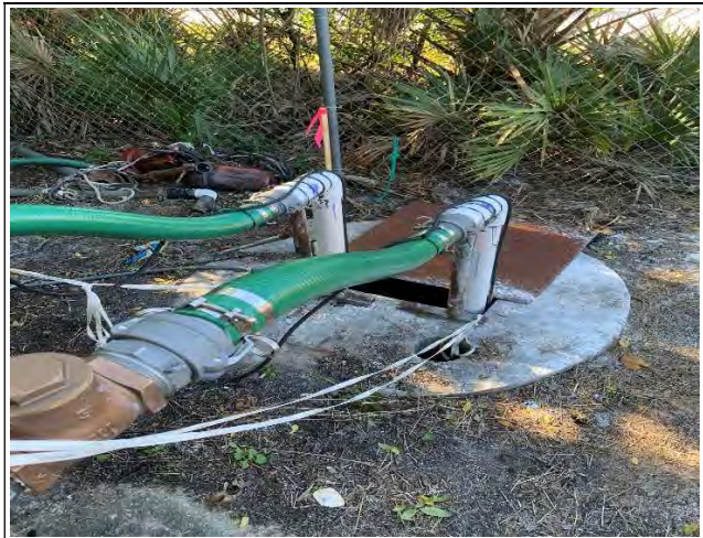
32. Lift station temporary pumps
