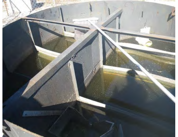
14 Chlorine contact chamber
