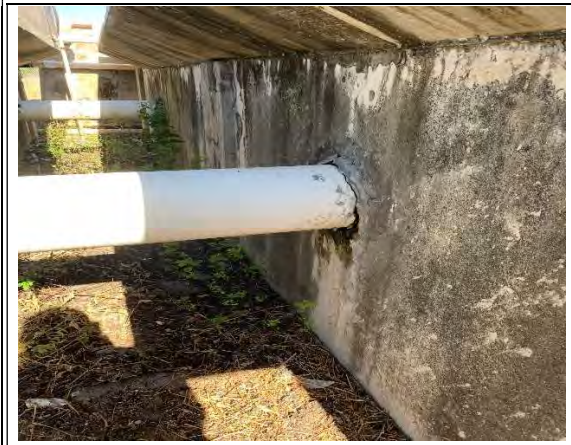
5. Leak coming from pipe entrance
