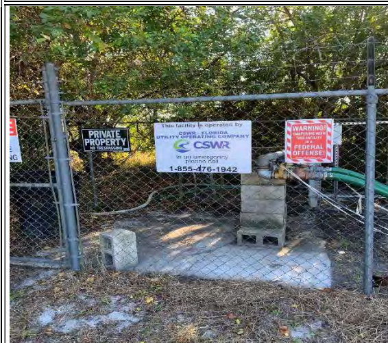
29. Signage on lift station
