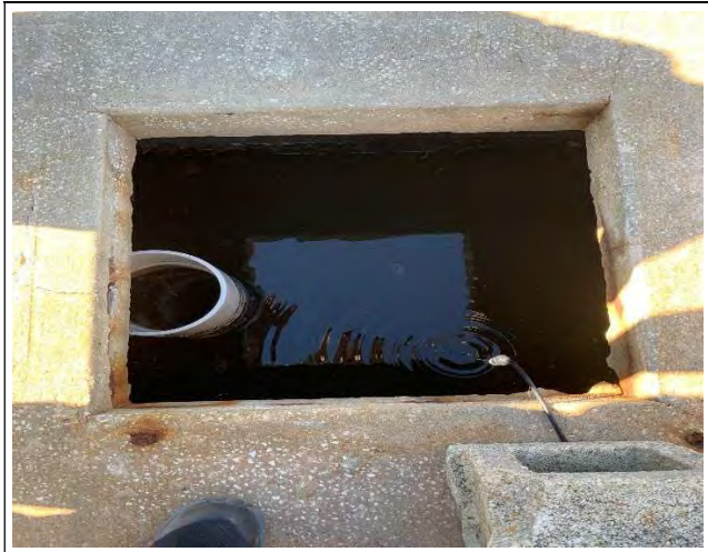
22. Chlorine Contact Chamber
