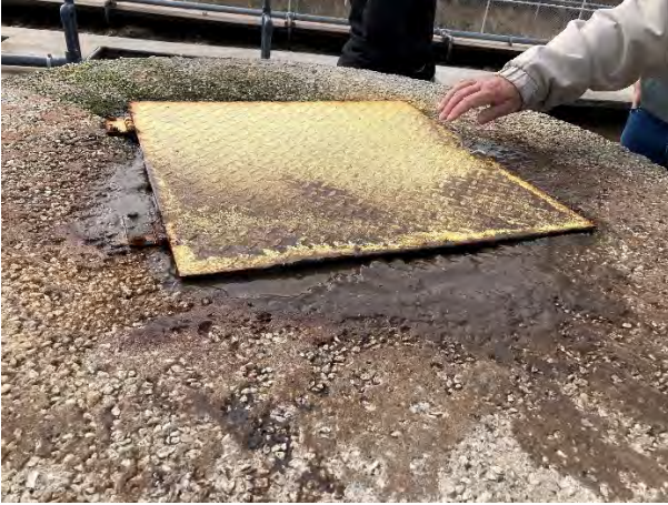
19. Sludge Holding Tank
