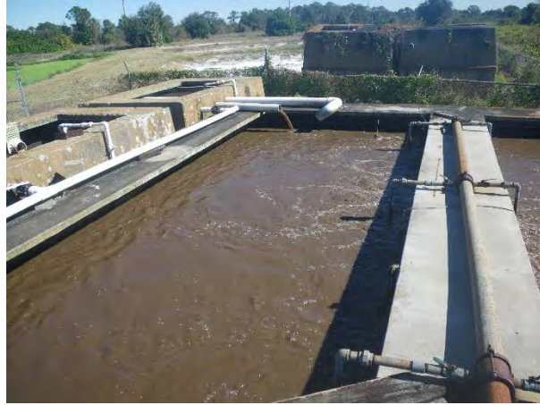
8 Fourth aeration basin and digesters
