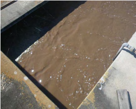
9 Dead spot at diffuser in third basin
