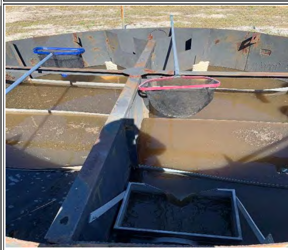
23. Chlorine Contact Chamber
