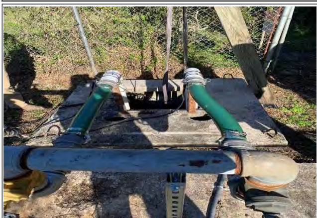
36. Lift station temporary pumps
