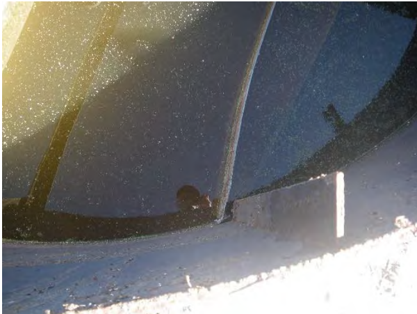
15 Separated baffle in CCC
