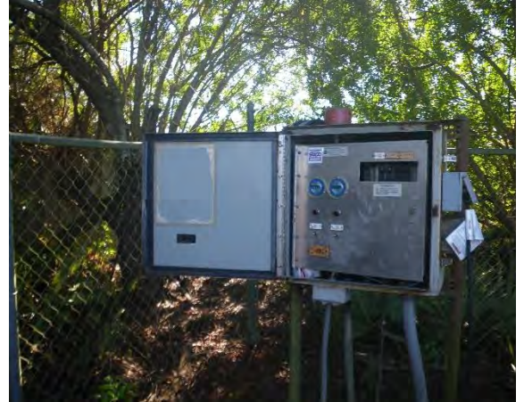
20 Clam Dr. electrical box
