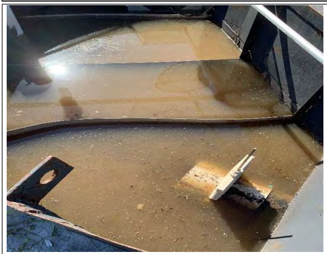
24. Chlorine Contact Chamber
