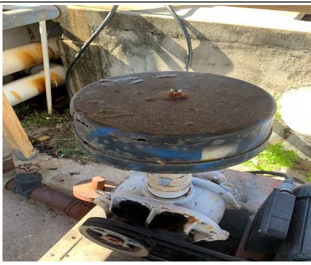
4. Rusted motor cover
