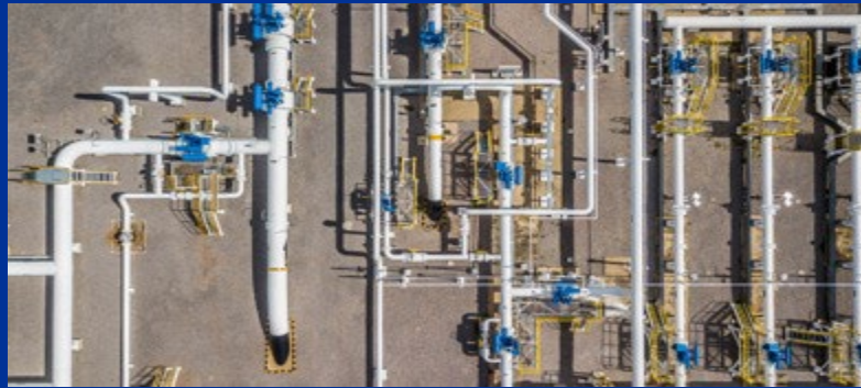
Existing Natural Gas Pipeline through Blending and/or New Infrastructure
