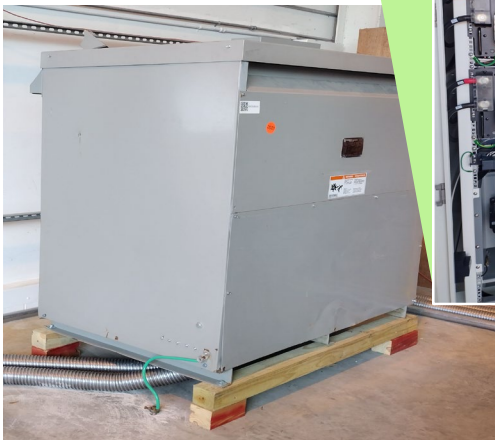
Step up Transformer: 500 KVA (480 V/600V)
