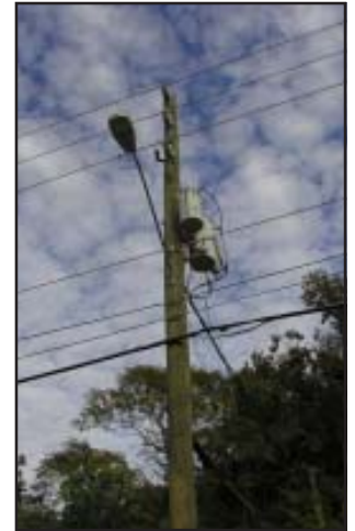
The Commission required the electric investor-owned utilities to provide support for their wood pole inspection plans.
