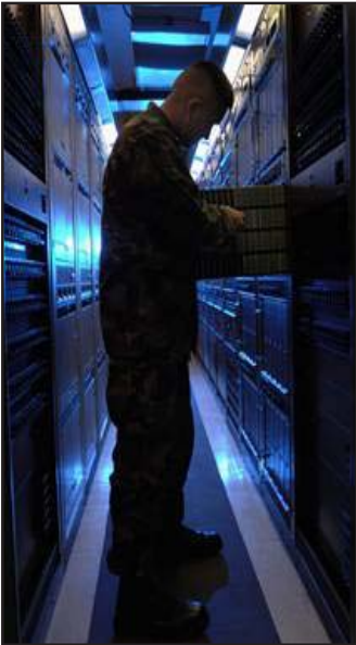
Commission staff evaluates the quality of service provided by telecommunications companies and conducts periodic on-site inspections of telecommunications facilities.
