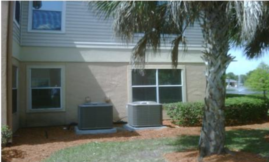
Picture of new SEER 15 Heat Pumps installed and new Window Film.
