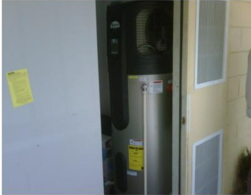
Picture of new Water Heater Heat Pump.
