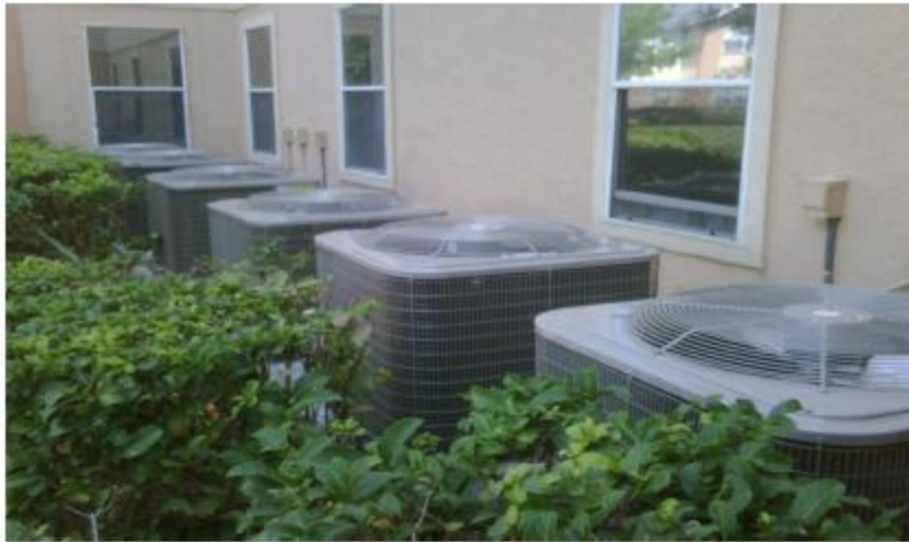
Picture of new SEER 15 Heat Pumps and Window Film
