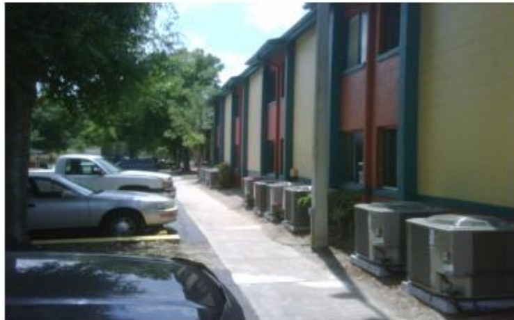
Picture of the new SEER 15 heat pump condenser units.
