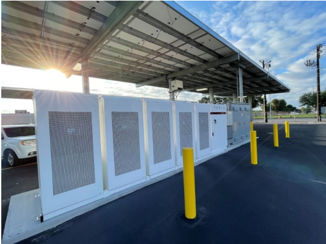
(North end of IRES carport solar array, with commercial batteries)
