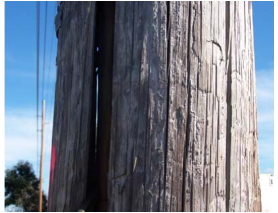
State 5 Pole Shell Crack
