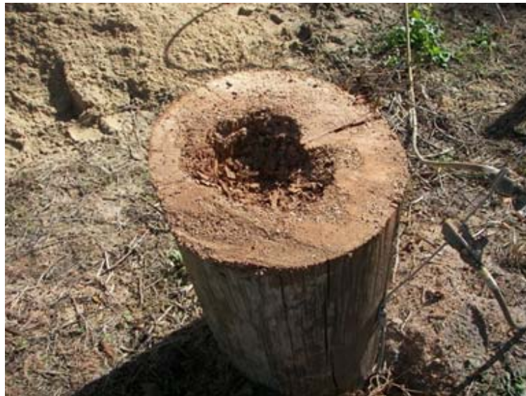
State 4 Pole w/ Internal Decay
