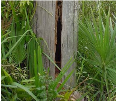
State 5 Shell Crack
