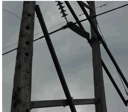
Priority 1 Groundline Pole Decay (with large internal cavity)
