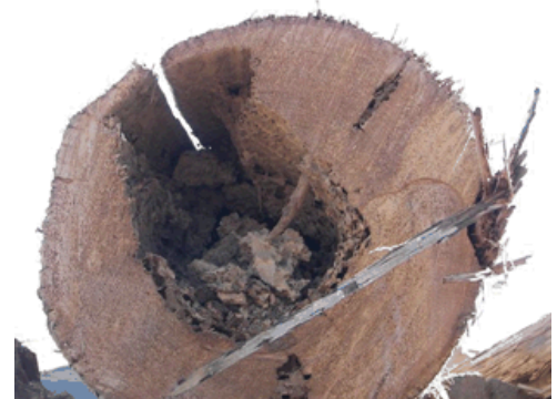
Priority 1 Internal Decay (Deep decay pocket)
