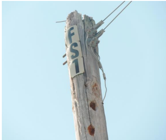
Priority 2 Split Pole Top & Vertical Woodpecker Holes
