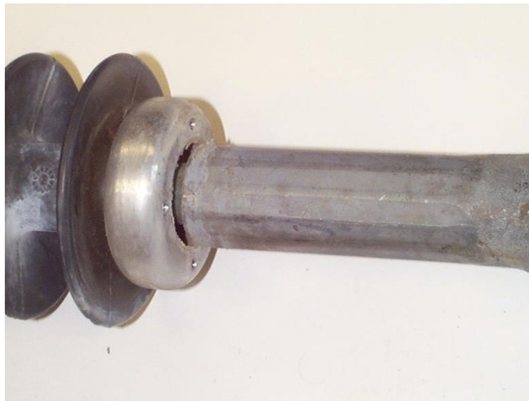
Priority 2 Polymer Insulator Exposed Fiberglass Rod (Ohio Brass)
