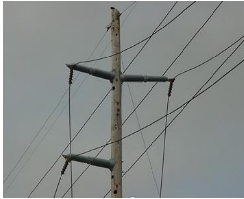
Priority 2 Woodpecker Holes (located in critical spots)
