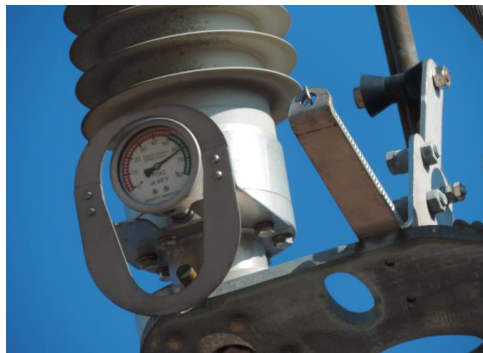
SF6 Gas Level on Southern States must be in the Green Region
