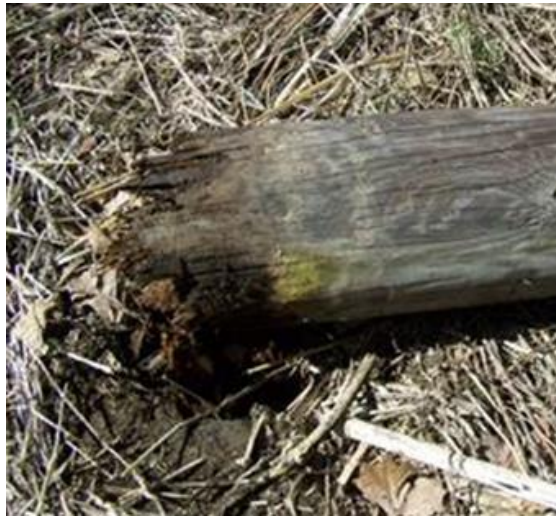
Green Growth (May be an indicator of substantial pole decay)
