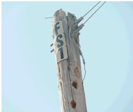
Priority 2 Split Pole Top & Vertical Woodpecker Holes
