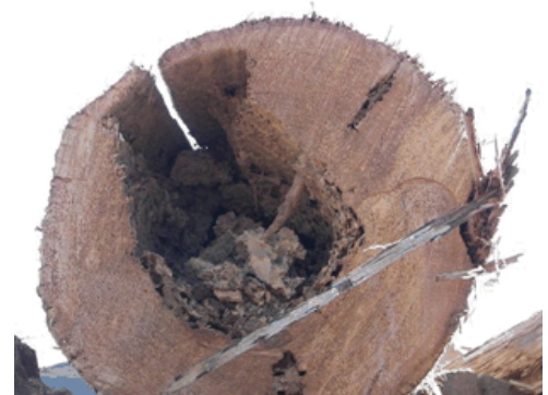
Priority 1 Internal Decay (Deep decay pocket)
