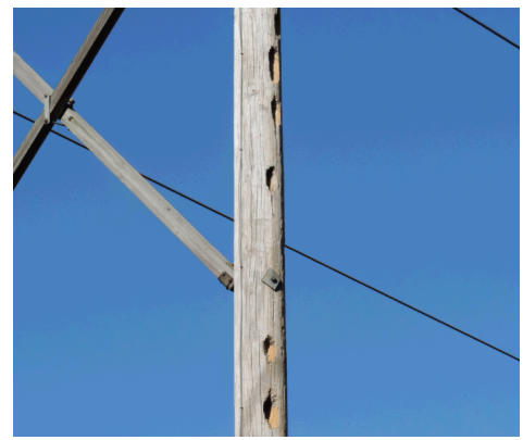
Priority 2 Woodpecker Holes (Quantity and orientation indicates significant pole decay)
