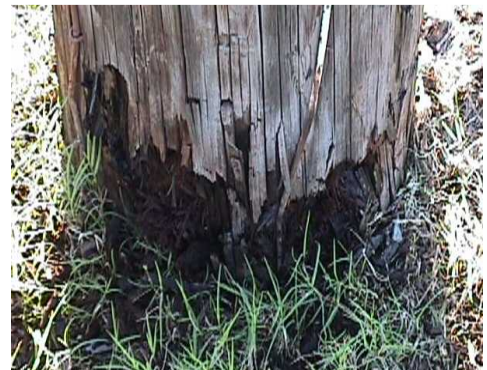
Priority 1 Groundline Pole Decay
