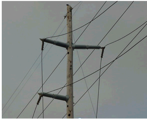
Priority 2 Woodpecker Holes (located in critical spots)
