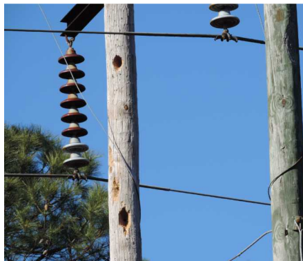
Priority 9 Woodpecker Holes (Not in critical locations)
