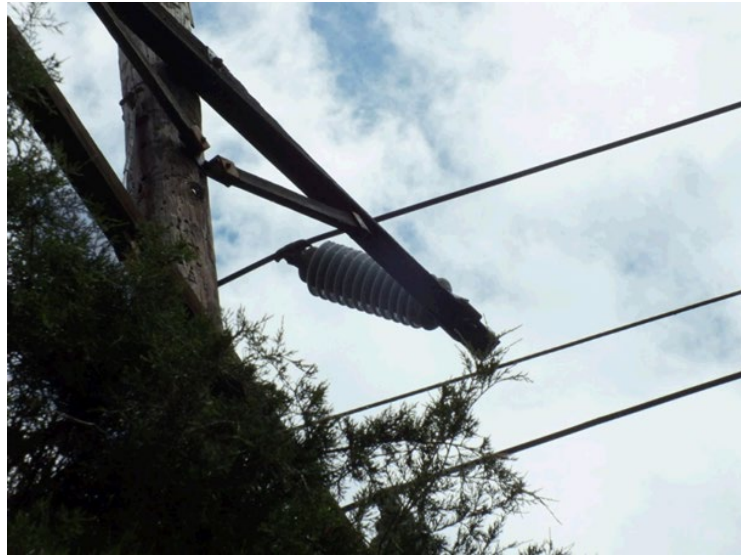
Priority 2 – Rolled pin insulator greater than 30 degrees
