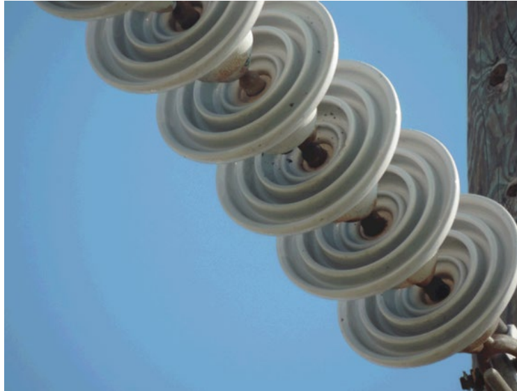
Priority 1 “Ball and Socket” insulator pin erosion
