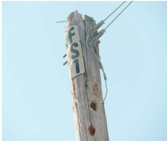
Priority 2 Split Pole Top & Vertical Woodpecker Holes
