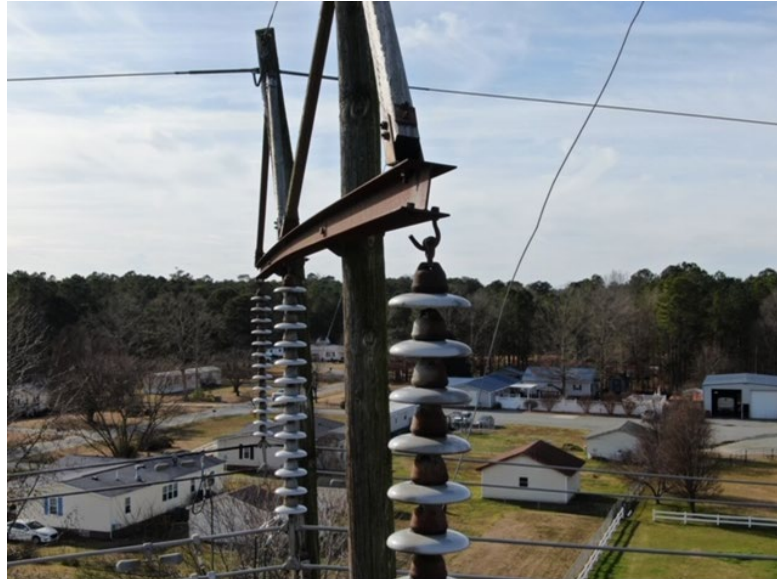
Priority 0 – Failed U-bolt detached on one end.
