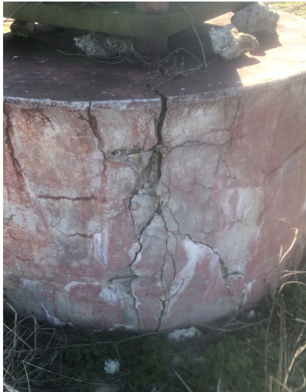
Priority 2 – Concrete foundation with cracking greater than ¼”
