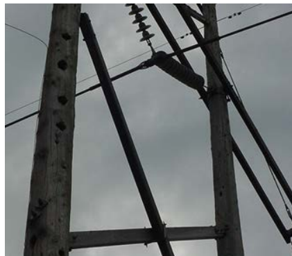
Priority 1 Woodpecker holes with a large internal cavity
