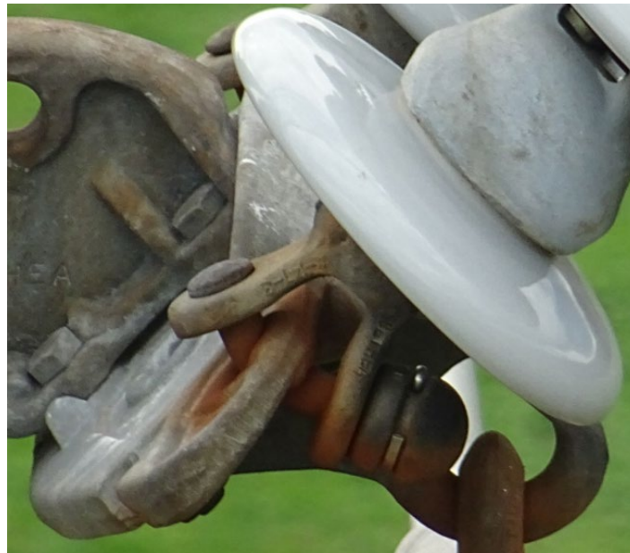
Priority 1 – Heavily rusted hardware suspected of wearing through pin.
