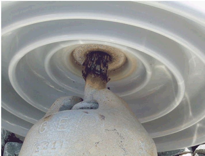
Priority 1 "Ball and Socket" insulator pin erosion
