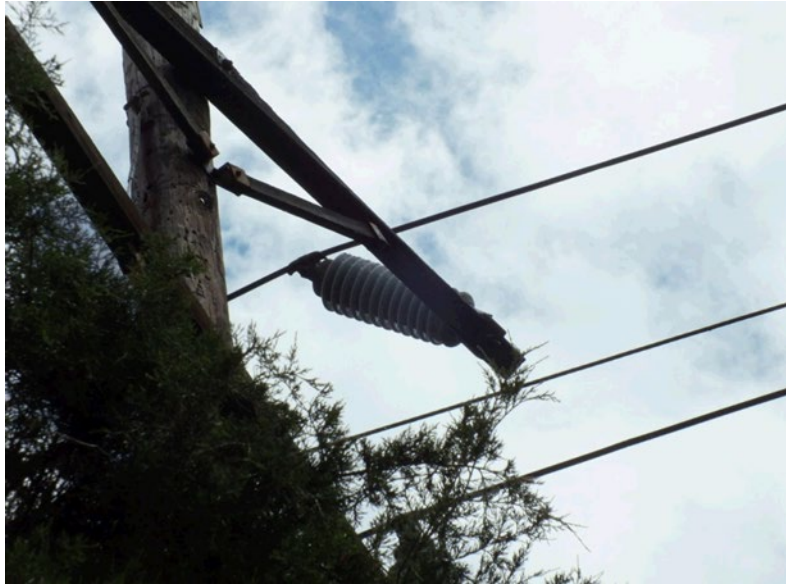
Priority 2 – Rolled pin insulator greater than 30 degrees
