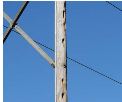
Priority 2 Woodpecker Holes (Quantity and orientation indicates significant pole decay)
