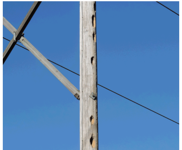
Priority 2 Woodpecker Holes - Quantity & orientation indicates significant decay
