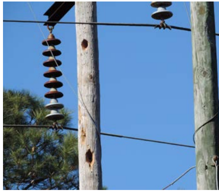
Priority 9 Woodpecker Holes (Not in critical locations)
