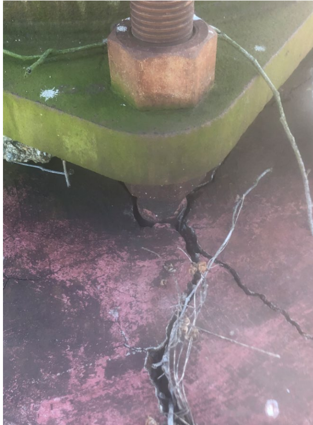
Priority 1 – Concrete foundation with cracks greater than ¼” and exposed anchor rods
