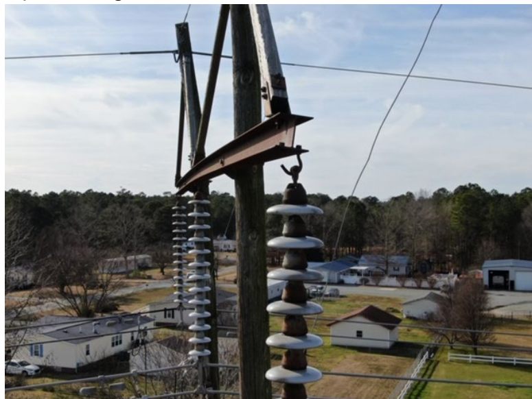
Priority 0 – Failed U-bolt detached on one end.
