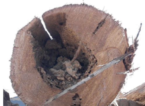
Priority 1 Internal Decay (Deep decay pocket)
