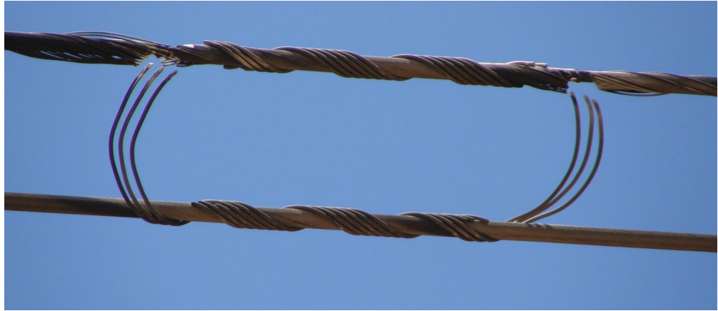
Priority 1 broken “Hair-pin” with >20% broken strands. Viewed from the ground.
