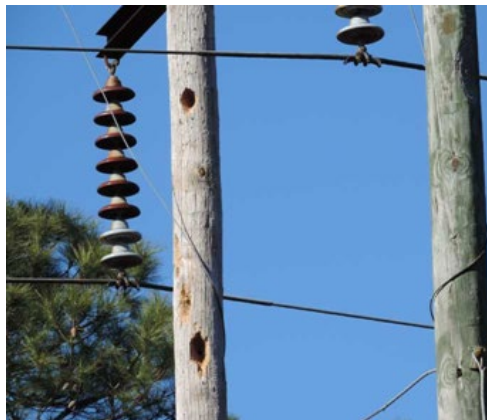
Priority 9 Woodpecker Holes (Not in a critical location)
