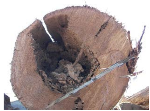
Priority 1 Internal Decay (Deep decay pocket)
