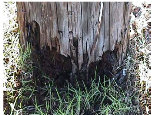
Priority 1 Groundline Pole Decay
