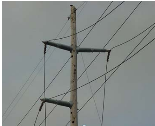
Priority 2 Woodpecker Holes (located in critical spots)
