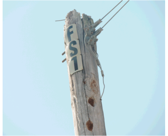
Priority 2 Split Pole Top & Vertical Woodpecker Holes
