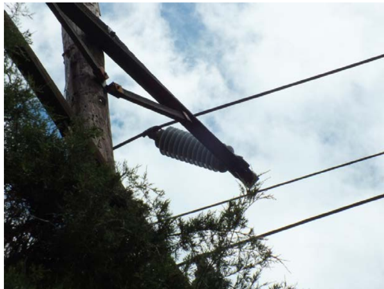
Priority 2 Rolled Pin Type Insulator Mounted above Wood Arm
