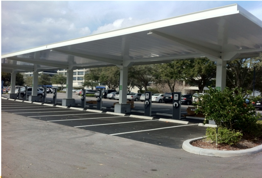
Solar carport at NextEra Energy HQ, Juno Beach, Florida
