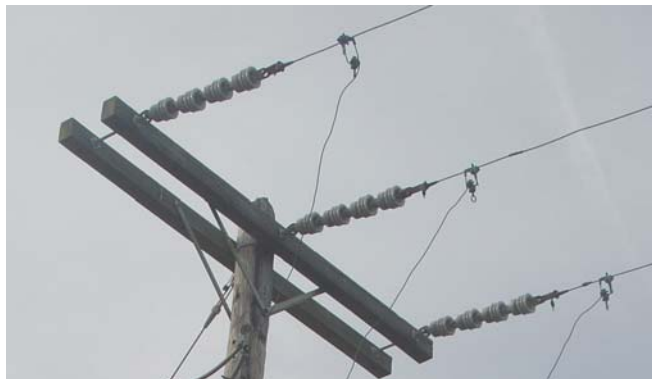
Overhead insulators along Blue Heron Blvd
