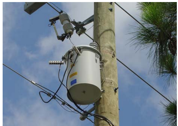
Overhead transformer along S. Jenkins Rd.
