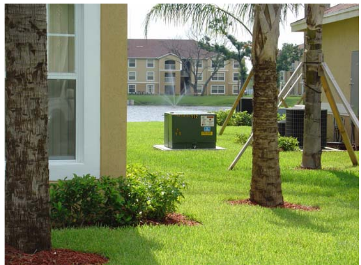
Access to this transformer is limited.
