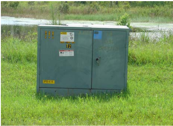
Easily accessible underground transformer
