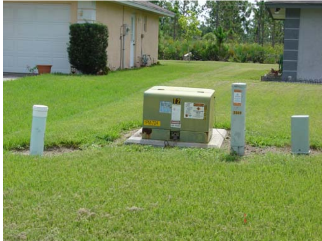
Underground congestion creates unpleasant scenery and possible touch potential issues
