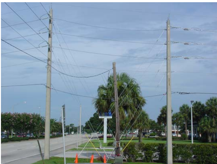
Guy wires on overhead lines can be hazardous to drivers
