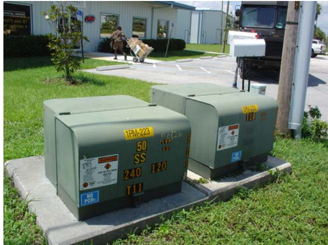
Padmount transformers close to roadways may be dangerous
