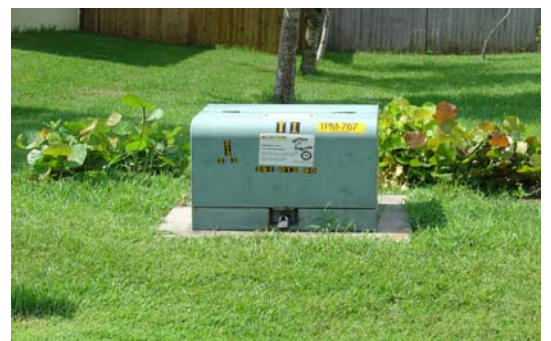
Padmount transformer in backyard
