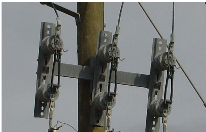
Solid blade disconnects on overhead line
