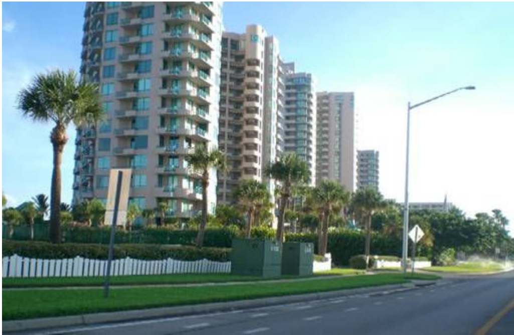
Figure 4-4. Pad Mounted Equipment on the Side of the Road in Sand Key
