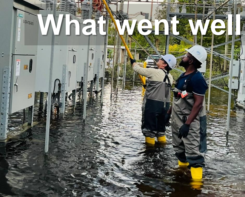
Substation Flood Monitors Mitigate Significant Damage
