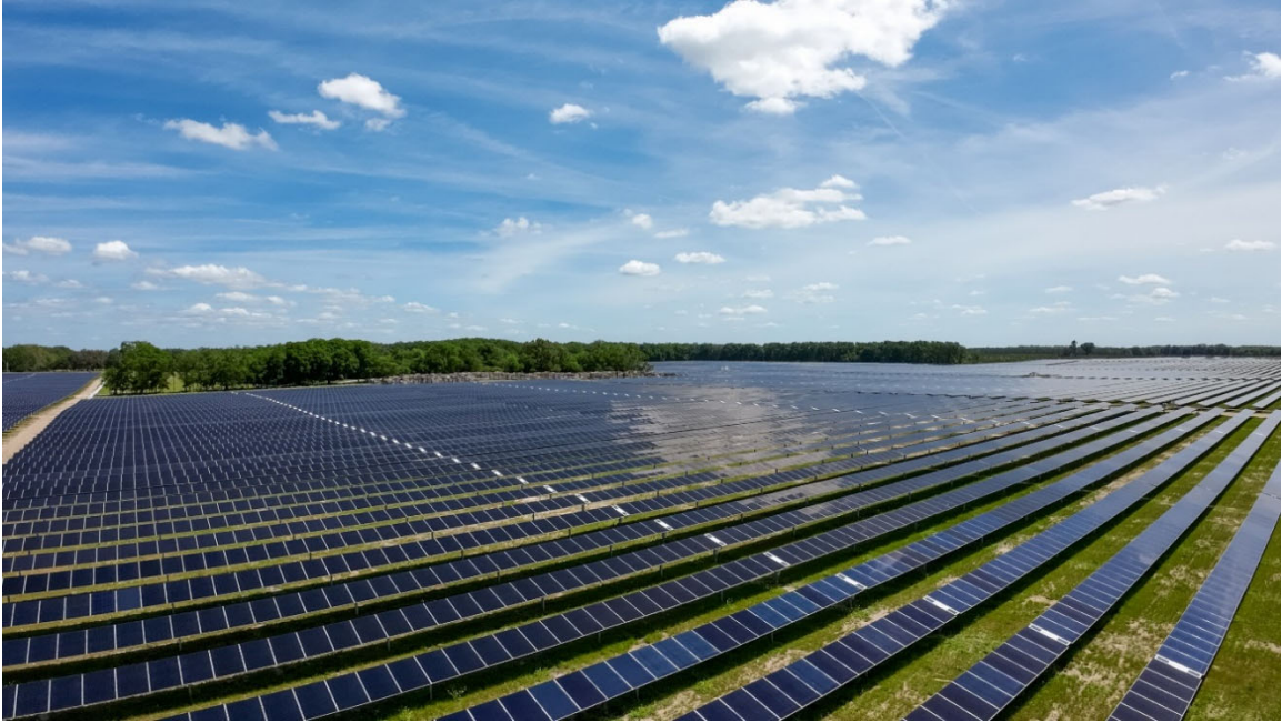
FIGURE 3.4 High Springs Solar Power Plant
