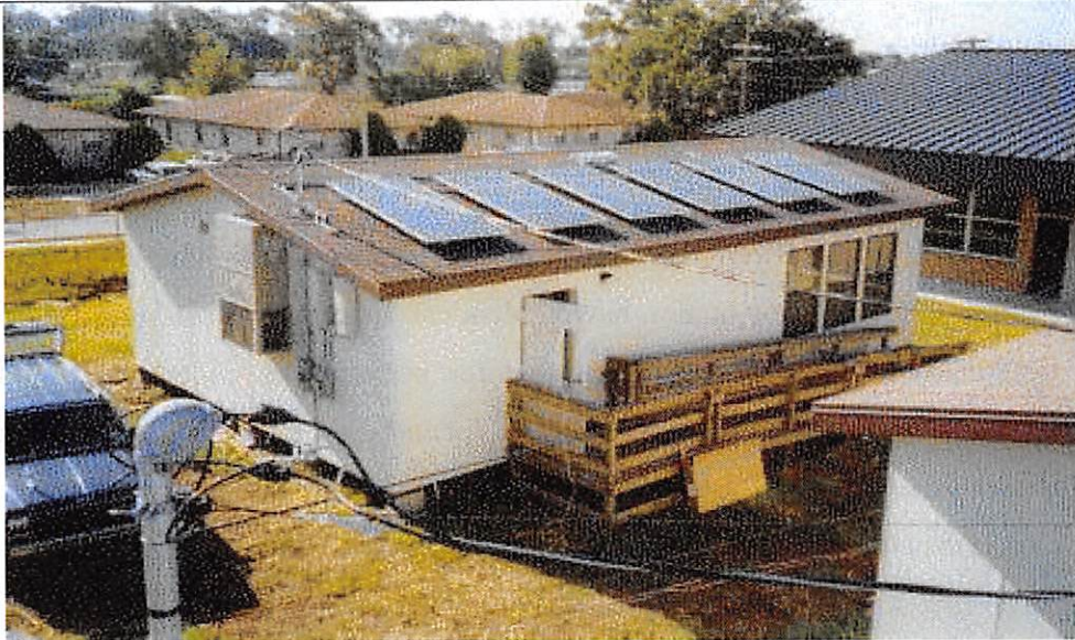
Figure 4-2 Portable Classroom Topped by PV Panels
