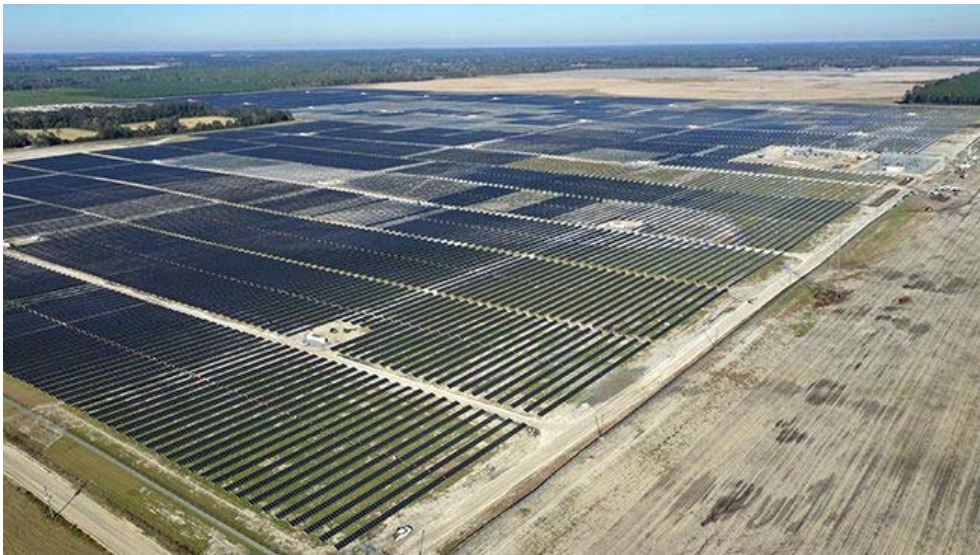
FIGURE 3.5 Hamilton Solar Site
