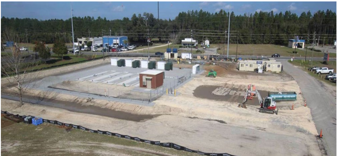
FIGURE 3.4 Trenton Battery Energy Storage System
