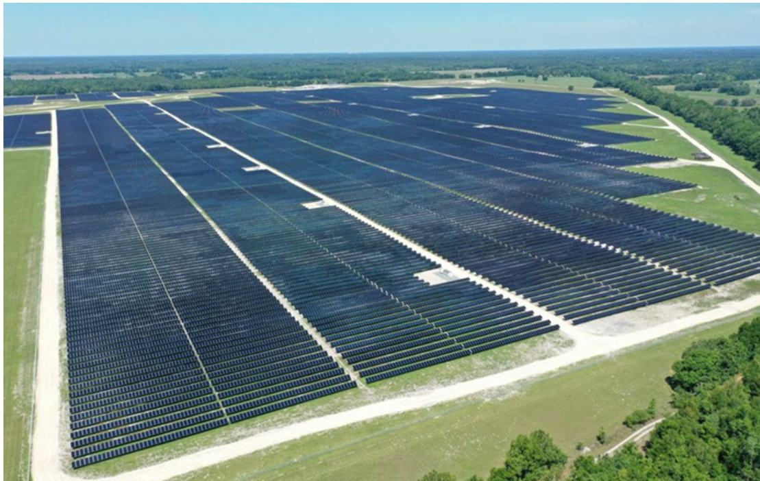
FIGURE 3.2 Santa Fe Solar Power Plant
