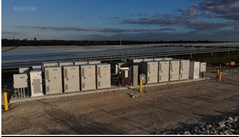
FIGURE 3.9 Lake Placid Battery Energy Storage System
