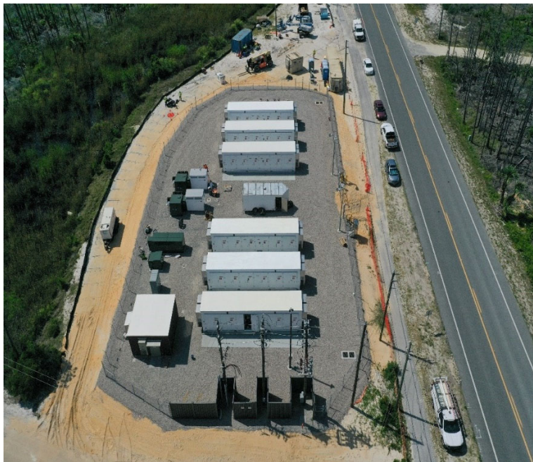
FIGURE 3.6 Cape San Blas Battery Energy Storage System
