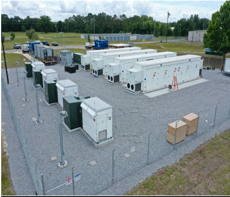
FIGURE 3.5 Trenton Battery Energy Storage System
