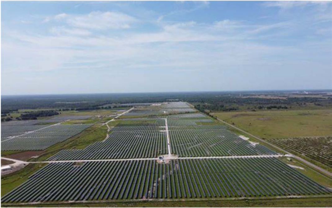
FIGURE 3.4 Charlie Creek Solar Power Plant
